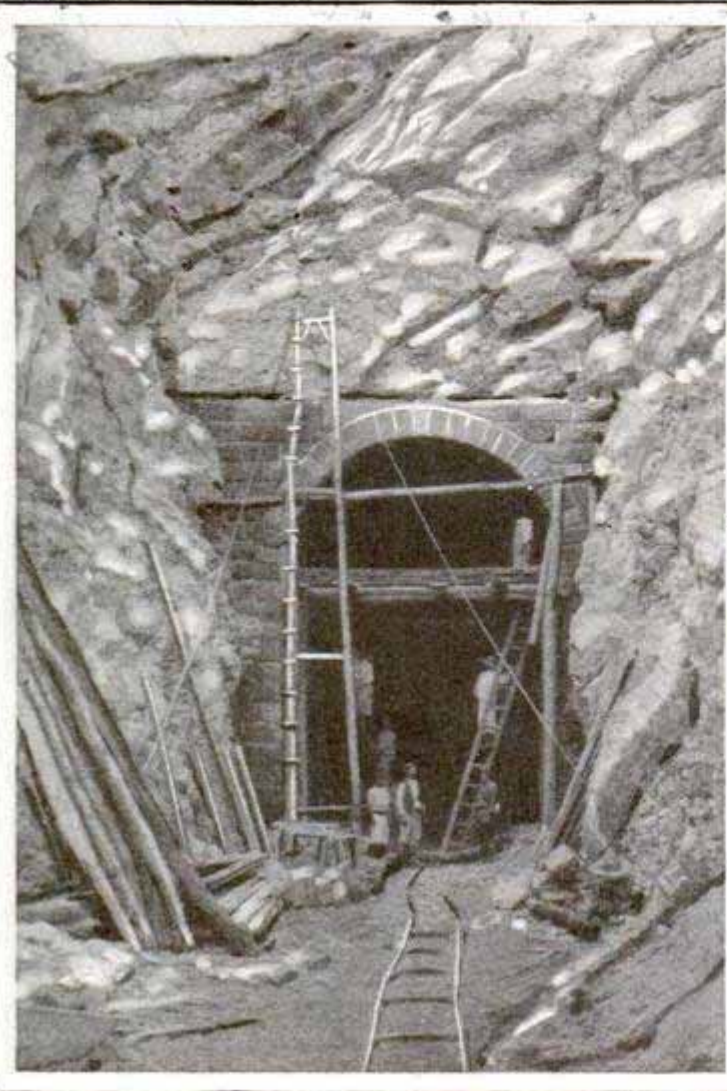
Tunnel Entrance on Miravelles River Section of Southern Pacific of Mexico; Masonry Is of Permanent Construction
