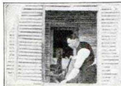
View of part of the interior of the bungalow for practicing house wiring—right in the Greer Shops. You learn here by real experience—with an expert always at hand to show you how.
