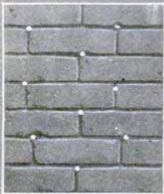
Roofers' Nails Hold Stucco to Old Wall
