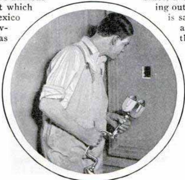
Cutter Used with Hand Brace, and Opening Made in Wall for Electric Switch
