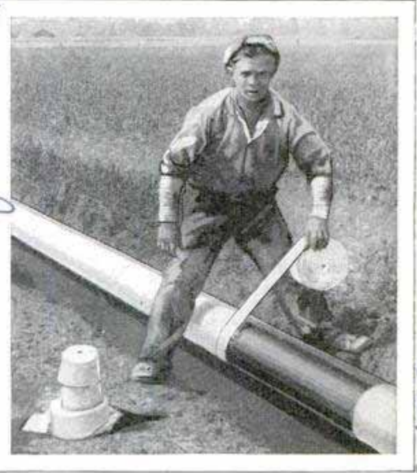
Embalming a Gas Main; This Expert Taper Can Cover a Twenty-Foot Length in Two Minutes
