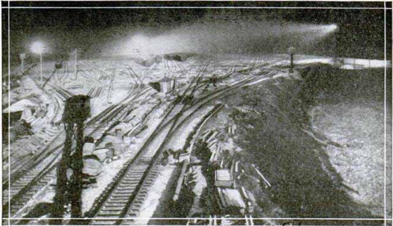
Big Railroad Yards Brilliantly Illuminated with Powerful Searchlights to Aid Night Work; Forty-Five Reflectors Are Used
