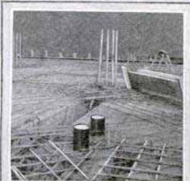
Stovepipes Set in Forms and Filled with Sand Provide Openings in Concrete Floor
