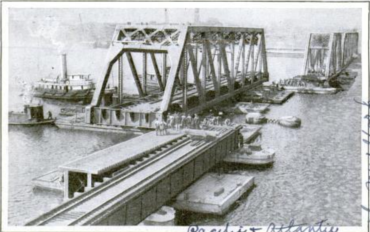
Rolling Bridge Span into Its Place upon Piers from Floating Barges, on Which It Was Towed After Old Span Had Been Removed; Both Jobs Required Only Six Hours
