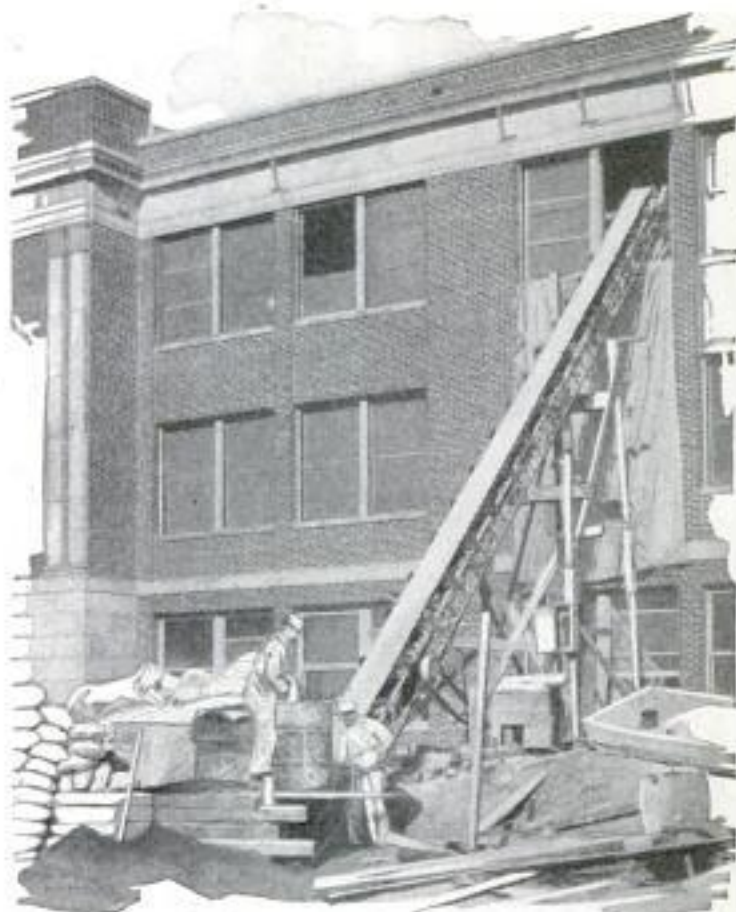
Conveyor Carries Plaster to Floors of Building to the Plasterers in Three Minutes
