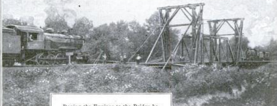
Roping the Engines to the Bridge before Lifting; the Wooden Uprights at Each End Formed a Track for the Structure
