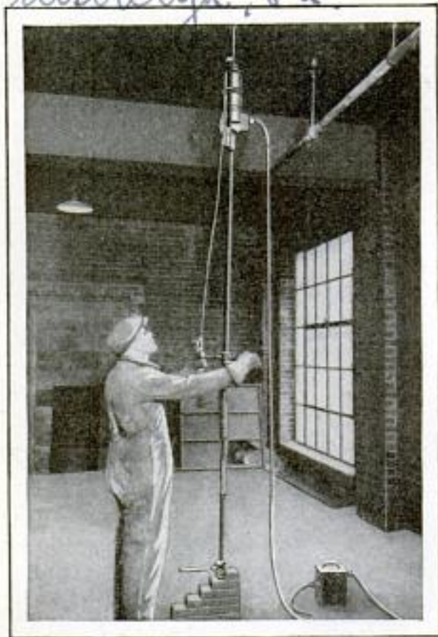
Boring Hole in Concrete Ceiling with Overhead Electric Drill on Telescoping-Tube Support
