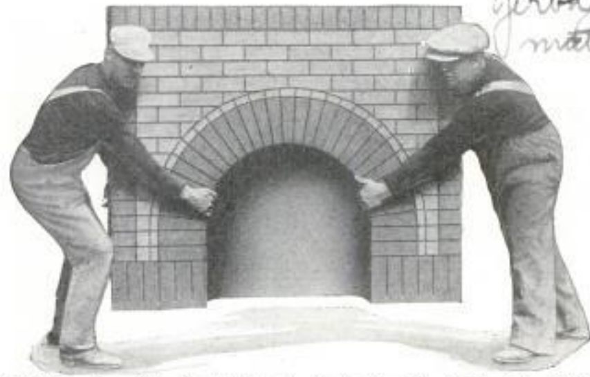
Installing One of the Portable Mantels; Its Surface Closely Resembles Brick and Patterns and Colors Can Be Harmonized with Interiors.
