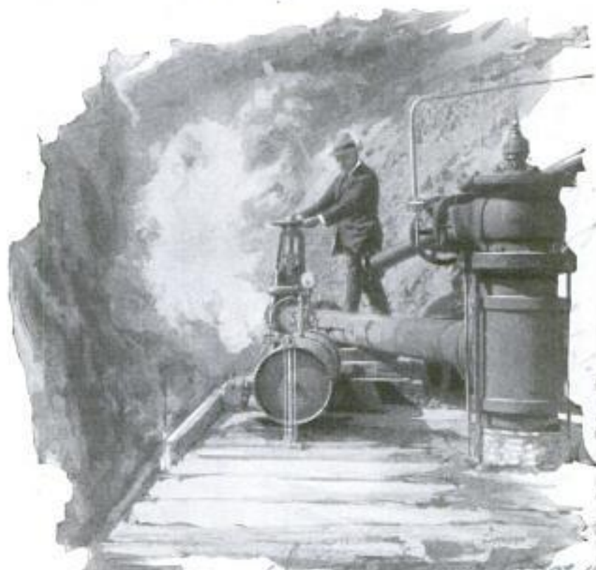
Roaring Up from Natural Boiler Below, Steam Is Trapped in These Pipes to Turn Dynamos
