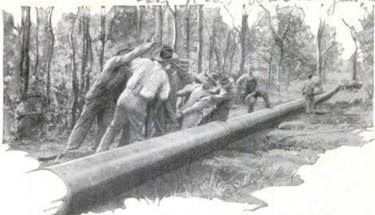
"Heave Ho!" and the "Bull Gang" Gives a Mighty Tug to Swing the Section Ends into Alignment
