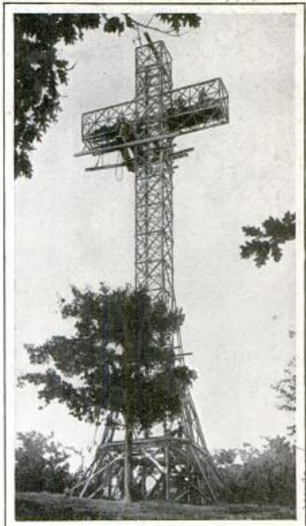
Finishing Steel Work on the Skyscraper Cross That Will "Preach" to Thousands Day and Night
