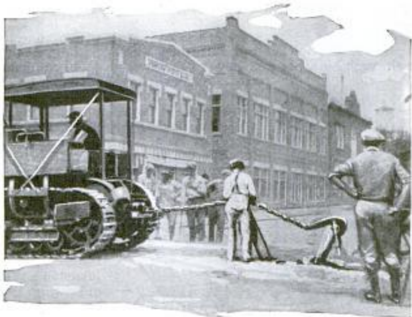
Breaking Up Old Concrete Pavement with Aid of Powerful Tractor and Hook
