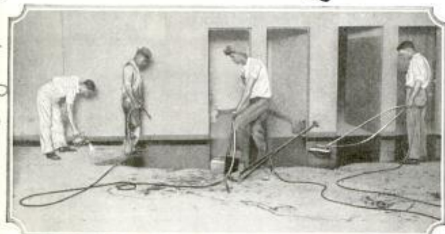
Waterproofing a Concrete Floor by Applying Composition and Treating It with Portable Electric Vulcanizer
