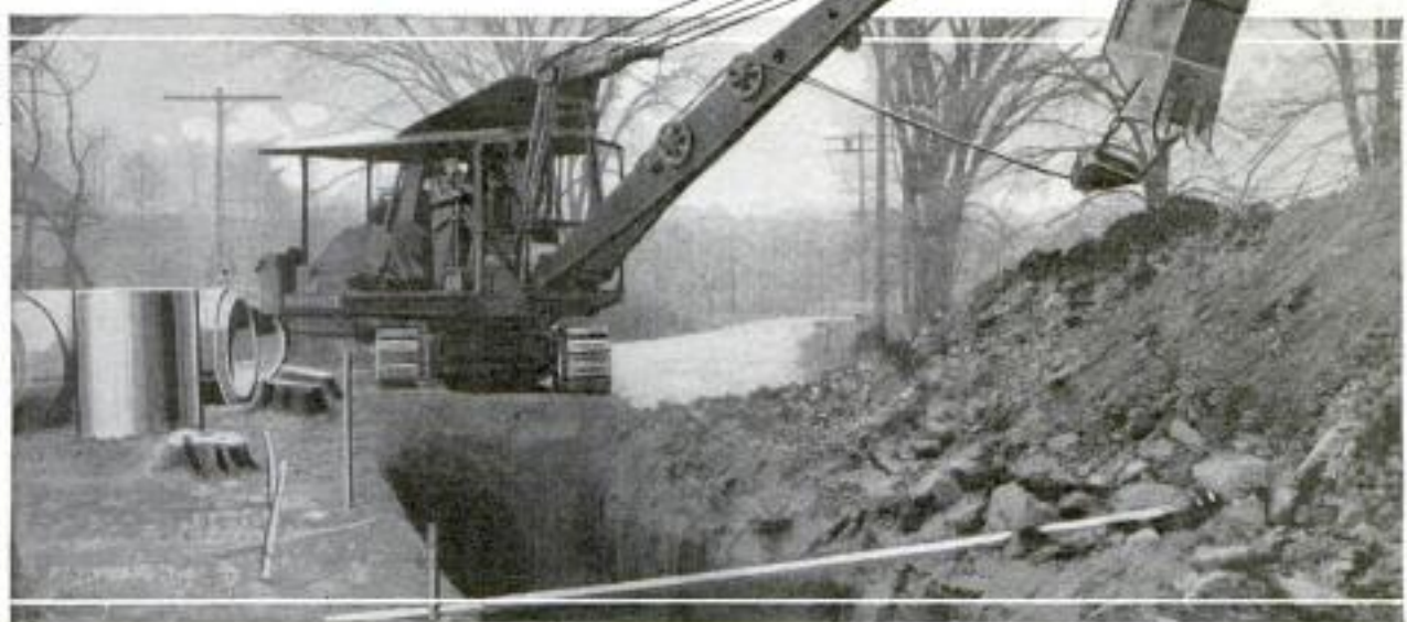
Trench Pull-Shovel Which Backs Away from Work, Needs No Mats and Never Has to Straddle the Trench; It Is Mounted on Crawler Treads and Driven by Gasoline Motor
