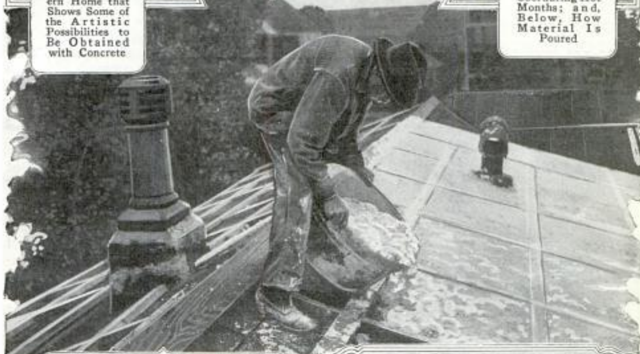
Slabs of Gypsum Used to Insulate Walls Being Cut and Placed between Studs after Material Has Been Poured on the Job and Has Partially Hardened.
