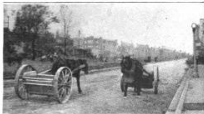
Driverless Horses which Have Been Trained to Carry Concrete Between the Mixer and the Dumps
