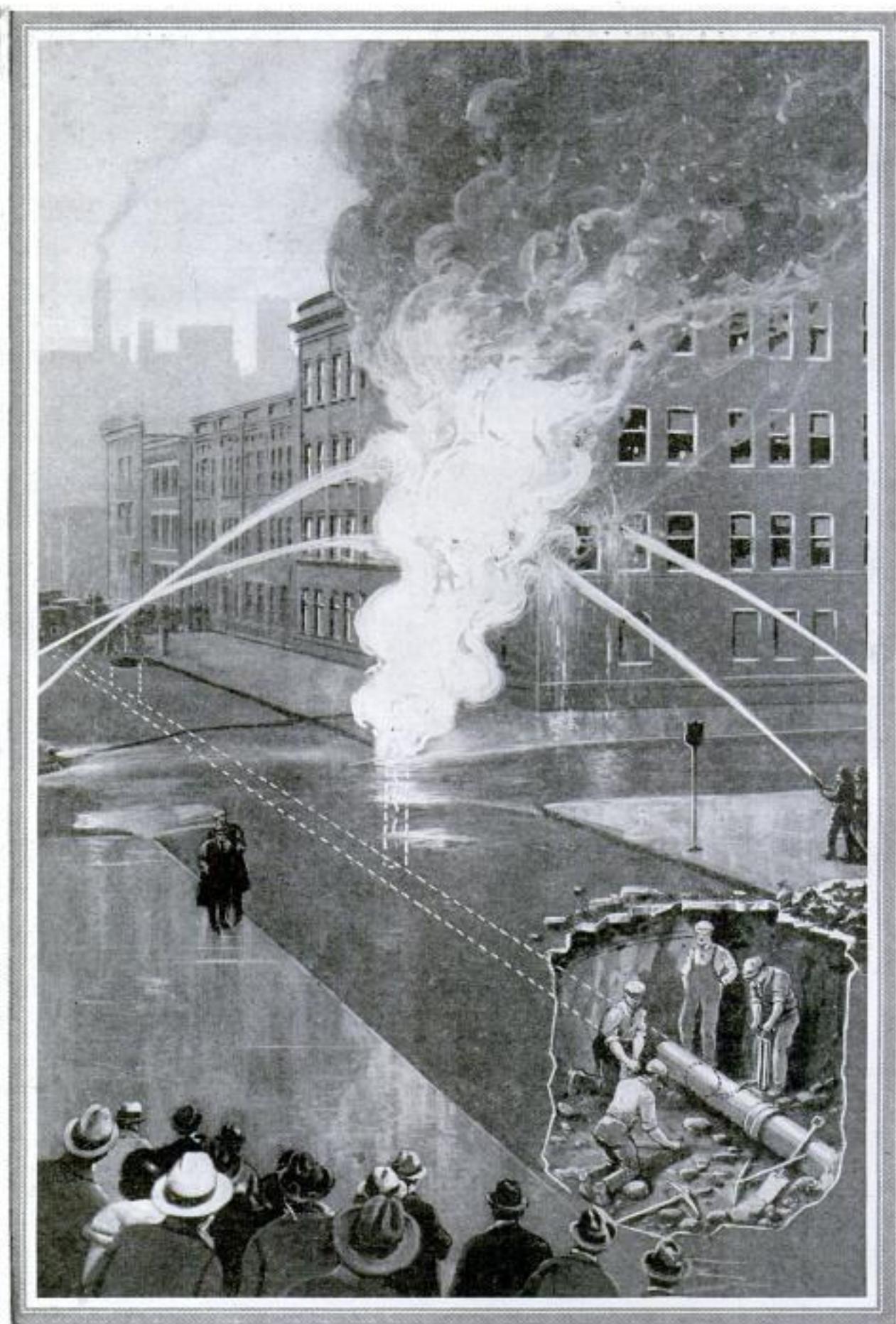
How Volcano of Flaming Gas from Leaking Street Main Was Conquered without Interrupting Service by "Plugging Off" a Section of the Pipe with Rubber Balloons—See Page 565.
