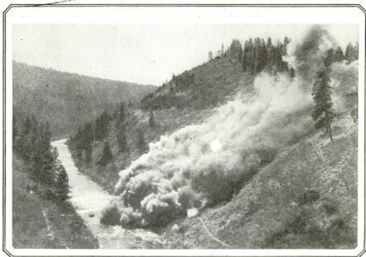
Tons of Earth Displaced on Mt. Shasta, California, to Make Way for Dam Site: Taken Two Seconds After Explosion Started, Picture Shows Its Downward Sweep
