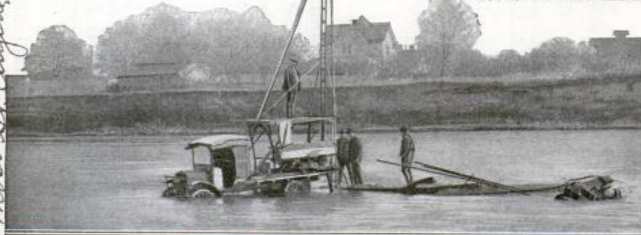
Drilling Down to Bedrock in the Willamette River to Determine the Necessary Depth for Caissons
