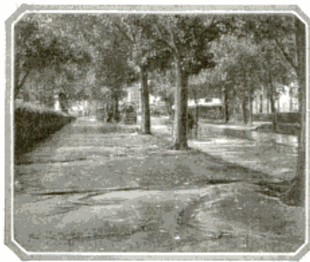
Street and Sidewalk Cracked by Shallow, Spreading Roots of the Popular Silver Maple
