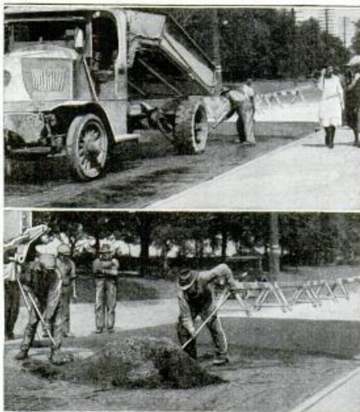
Above, Dumping the Heated Sheet Asphalt; Below, Spreading Pure Asphalt over the Old Pavement
