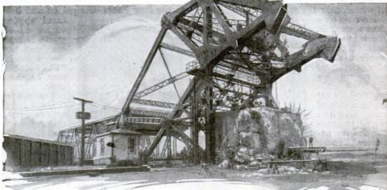
Heavy Concrete Balance Weight of Drawbridge which Crashed Down as the Great Span Was Being Lowered
