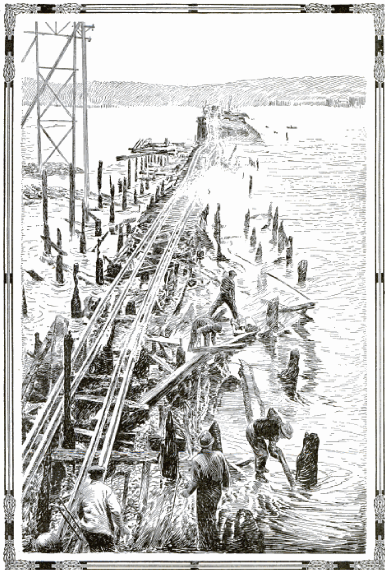
Reduced to a Mass of Charred Timbers and Twisted Metal by a Cascade of Flaming Oil, this Railroad Bridge Was Replaced in a Few Days' Time by Valiant Workers
