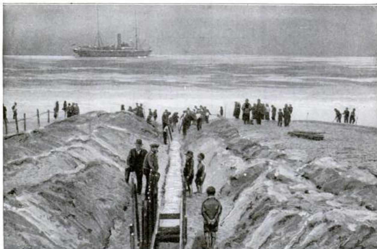
Pouring Concrete over the Shore End of the Cable and Its Guides to Hold Them Permanently to Their Moorings and to Protect Them from the Pounding Surf
