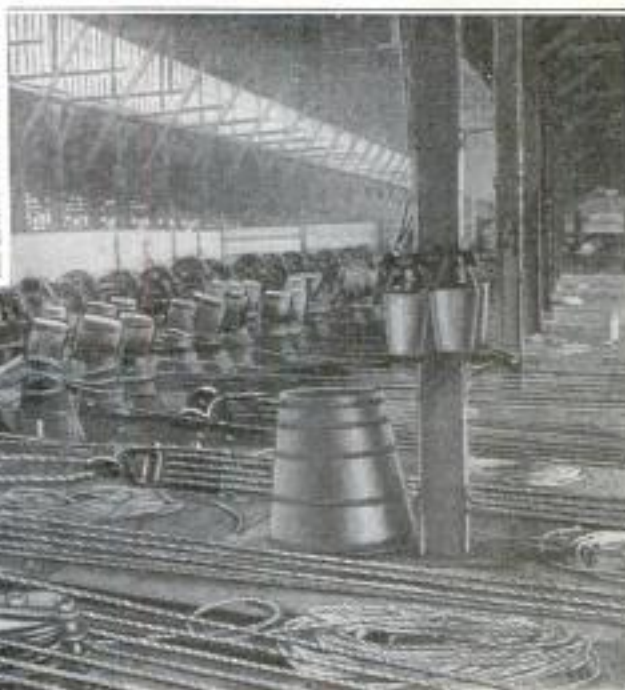
Twenty Winches and 132 Piles Driven into the Shore Served to Pull the Giant Hulk Upright. Above: Steel Structure on the Side of the Righted Hull
