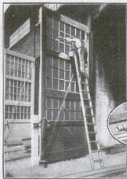
Dangerous reaching! It takes only a minute to re-set the ladder.
