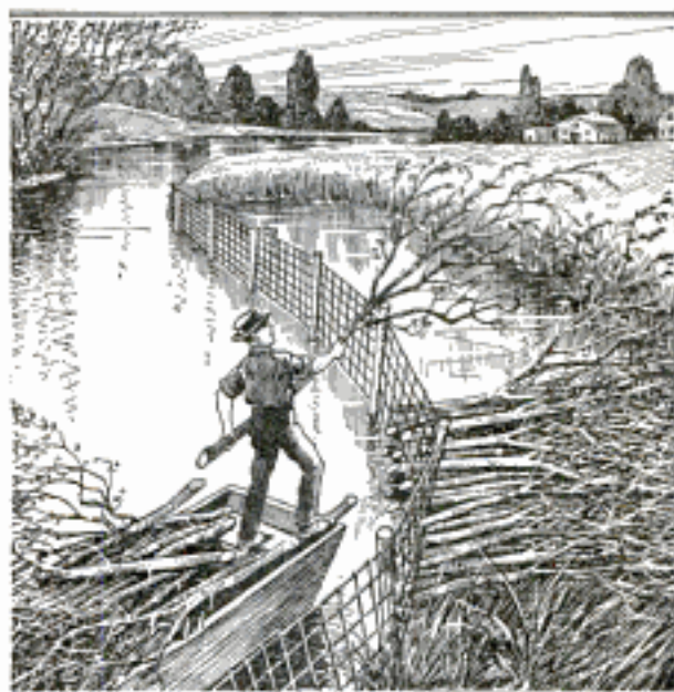
Method of Building an Inexpensive Wall to Prevent Erosion of Streams Having Low Banks
