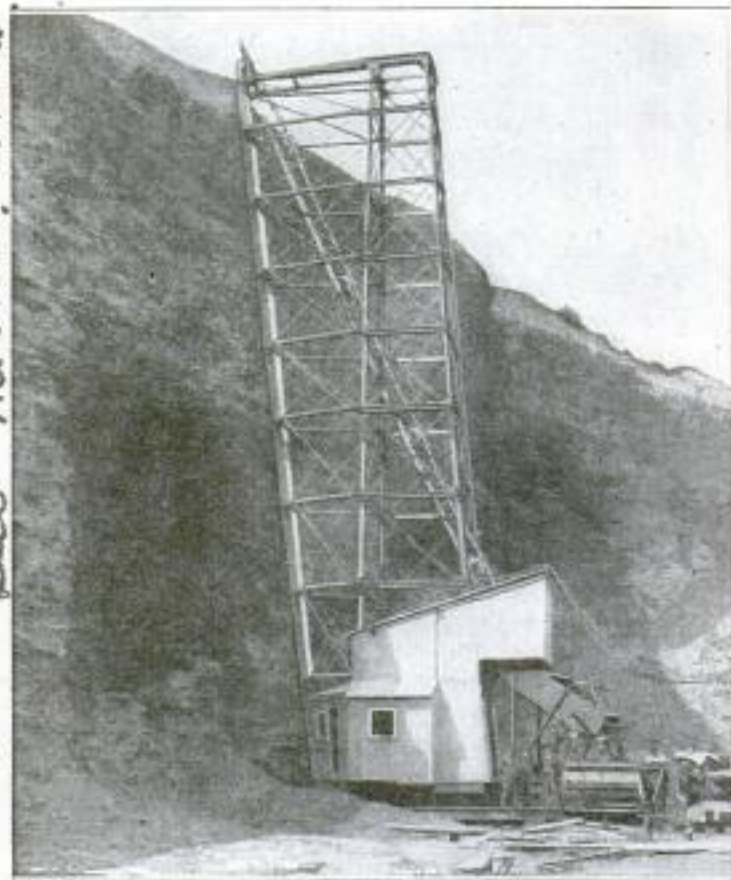
Tower for Scraping 50 Tons of Shale an Hour from Face of Cliff
