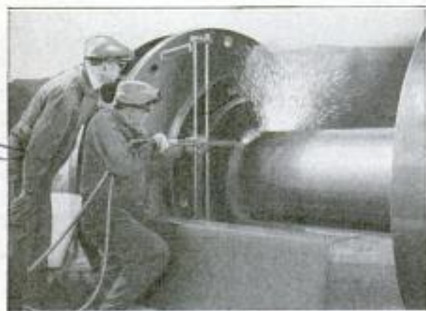
Cutting Through a 27-Inch Block of Steel with the Flame of Acetylene Torch
