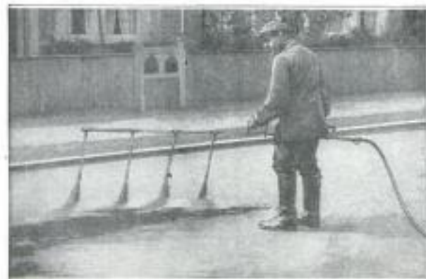
COPYRIGHT, CLARKE & HISE Hand-Pumped Spray for Spreading Tar Does Work of Four Men and Saves Material
