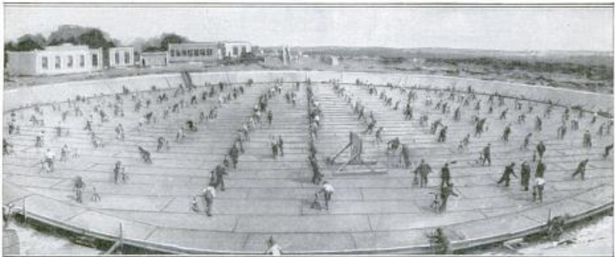
Lowering the Base of a Gas Tank in a Western City with 300 Men Using Small Hand Jacks: Forty Minutes were Required to Move This Tank, the Base Weight of Which Was 250 Tons
