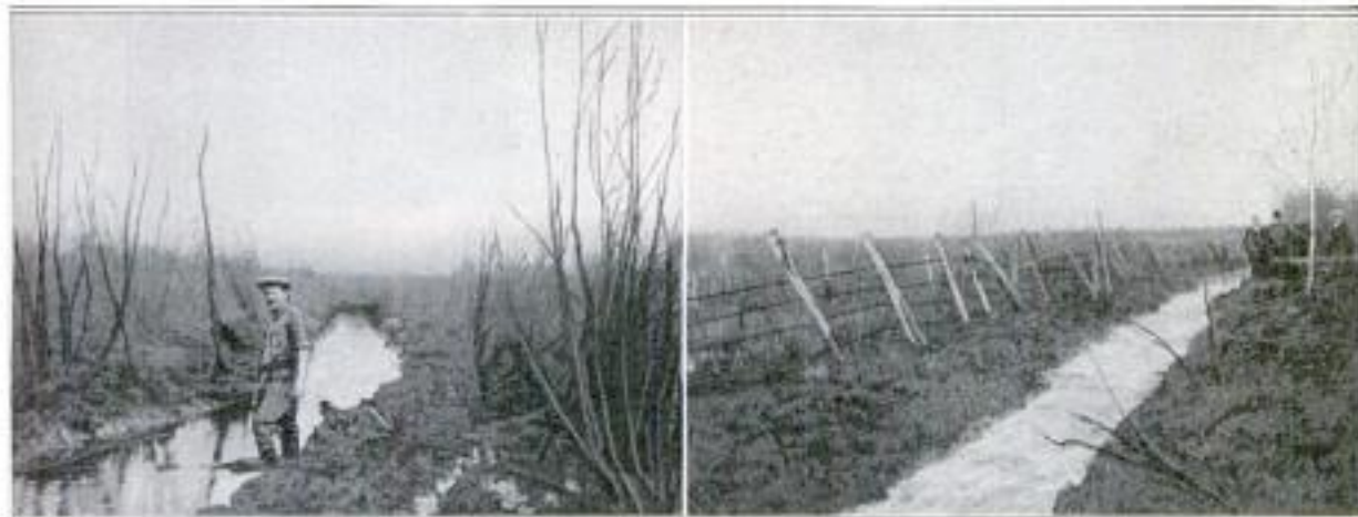
Left: Section of Ditch Blasted through a Swamp of Alder, Tamarack, and Cedar Trees. The Roots, Snags, and Stones Imbedded in the Wet Muck Offered Little Resistance. Right: Ditch Dynamited through Hardpan
