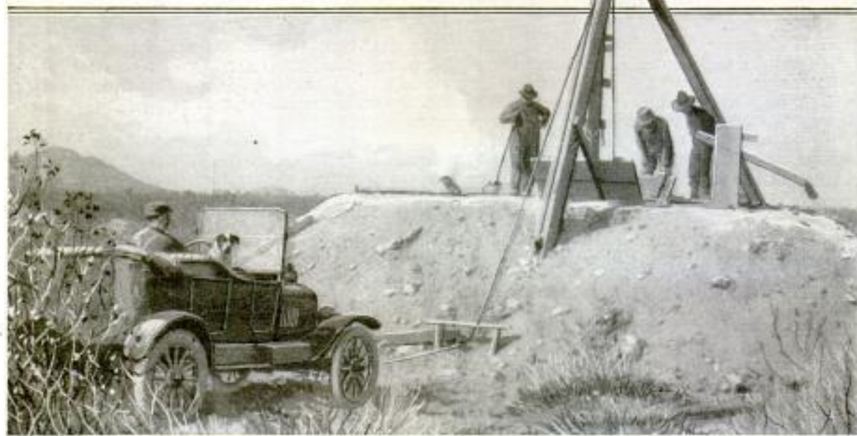
This View Illustrates the Resourcefulness of a Western Contractor, Who Used His Car for Hoisting Bucket Loads of Gold Out of a Shaft. The Method was Adopted After a Hand Windlass had been Tried and Found Wanting
