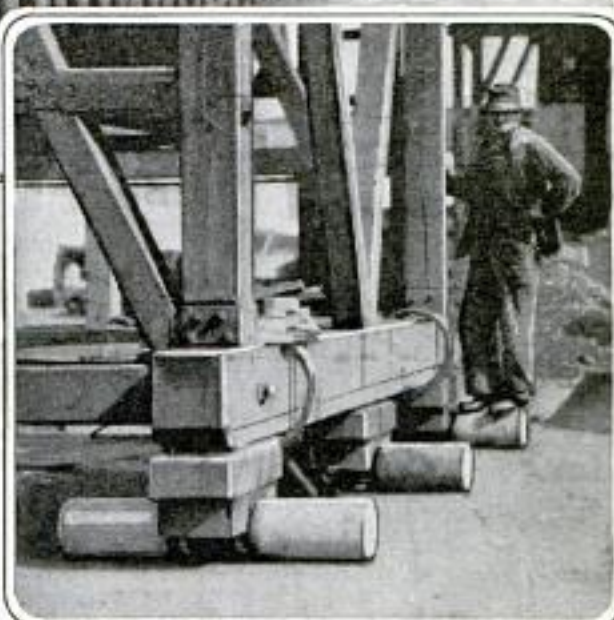
Close-Up of the Steel-Roller Bearings, of Which Six are Located under Each Coal Tower: Details of the Swivel Arrangement may Also be Seen
