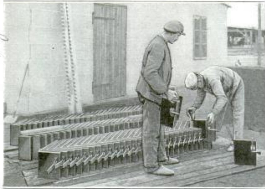
The German Method of Casting Building Blocks: Note the Economy of Placing the Forms So That the Blocks Have a Common Wall between Them
