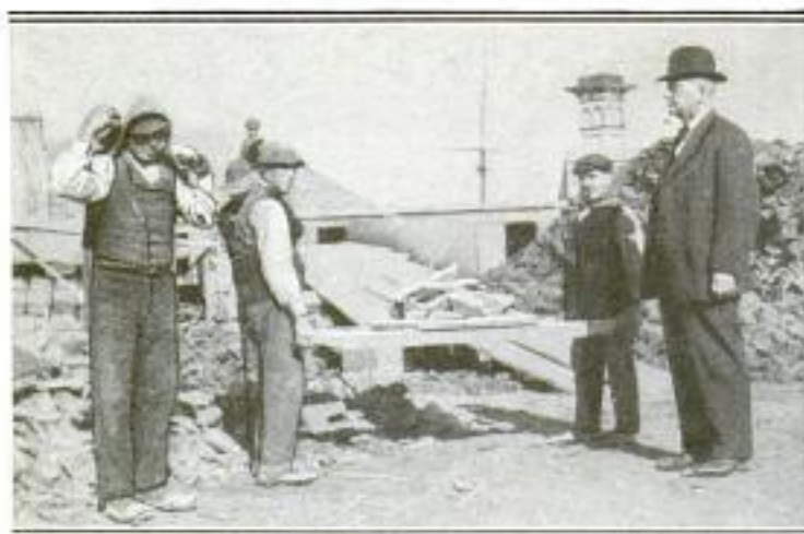
Two Workmen with a Litter Used in Carrying Rocks for the Building of the Hand-Constructed Packing Plant at the City of La Plata in Argentina
