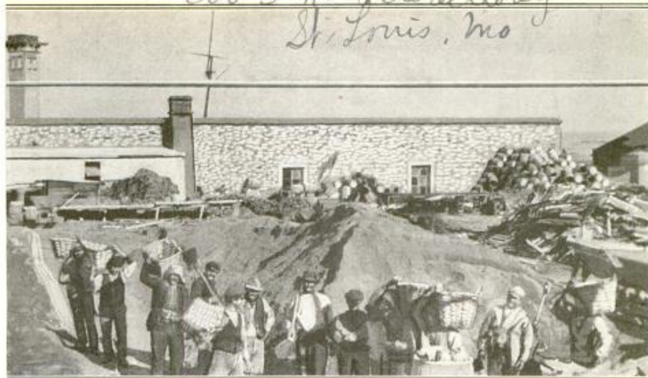
A Group of Argentinians with Baskets Which They Used to Transport Sand and Gravel to a Pit Where Concrete was Mixed for the Construction of a Packing Plant
