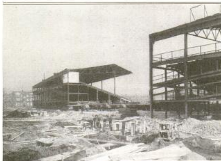
Close-Up of the Northwest Section of Stands after Moving, but before the New Box Seats were Added: Back of the Stand, at the Right, a Part of a Ramp Appears
