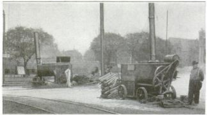
A Portable Repair Outfit for Pavement between, and Abutting, the Street-Car Tracks: The Sand and Asphalt are Heated to 400 and 370° Respectively before Mixing, the Higher Temperature of the Sand Keeping the Mix Sufficiently Hot to Flow Readily
