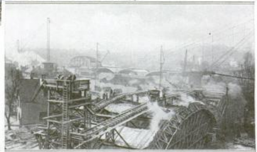
From the Tower, the Concrete-Filled Buckets were Hauled by Cable Out on Trestles Spanning the Arches, and Then Dumped at the Desired Points. The Bridge is to be Called the "Hill-to-Hill Bridge"
