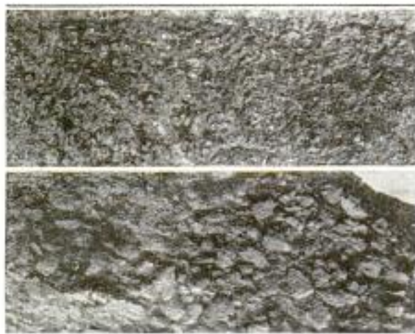
Above: Magnified Surface of Dense-Concrete Pile after Immersion in Sea Water. Below: Comparative View of Pile Made from Lean Concrete
