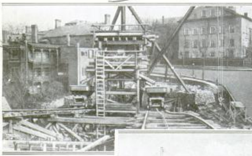
Tower at One End of the Bethlehem Bridge: After being Carried to the Top, the Concrete was Fed into the Buckets on Either Side
