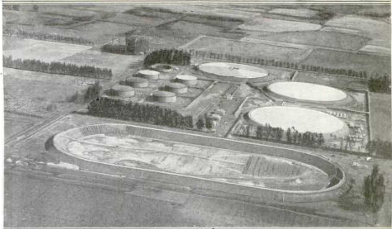
A Bird's-Eye View of the Mammoth 20-Acre Oil-Storage Tank under Construction, Which will Hold 1,750,000 Barrels of Oil When Completed: Its Roof will be Supported by Wooden Poles Set in Concrete Blocks in the Tank's Bottom. The Three Circular Tanks in the Background Are of 500,000-Barrel Capacity
