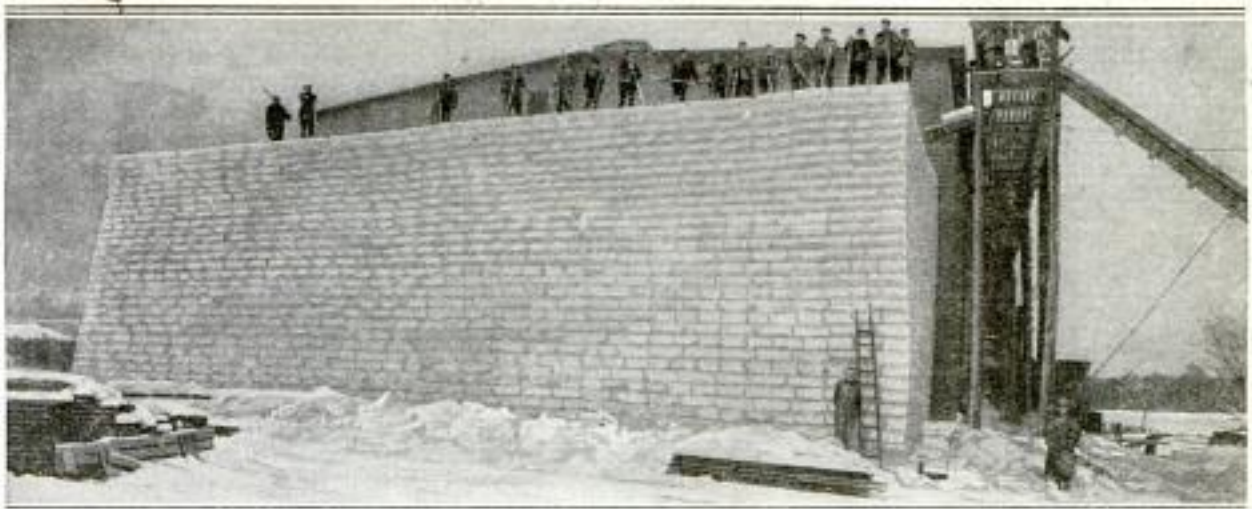
Building an Ice House around a Stack, 31 Feet High, with 10 Feet More to Go: A Prolonged Cold Spell Necessitated Storing This 3,000-Ton Pile Out in the Open, and the House was Subsequently Built over and around It
