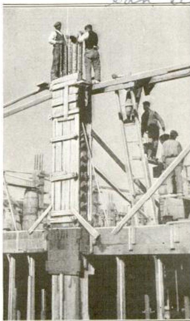
Argentinian Workmen Carrying Concrete in Buckets up a Ladder, and Pouring the Concrete into Forms
