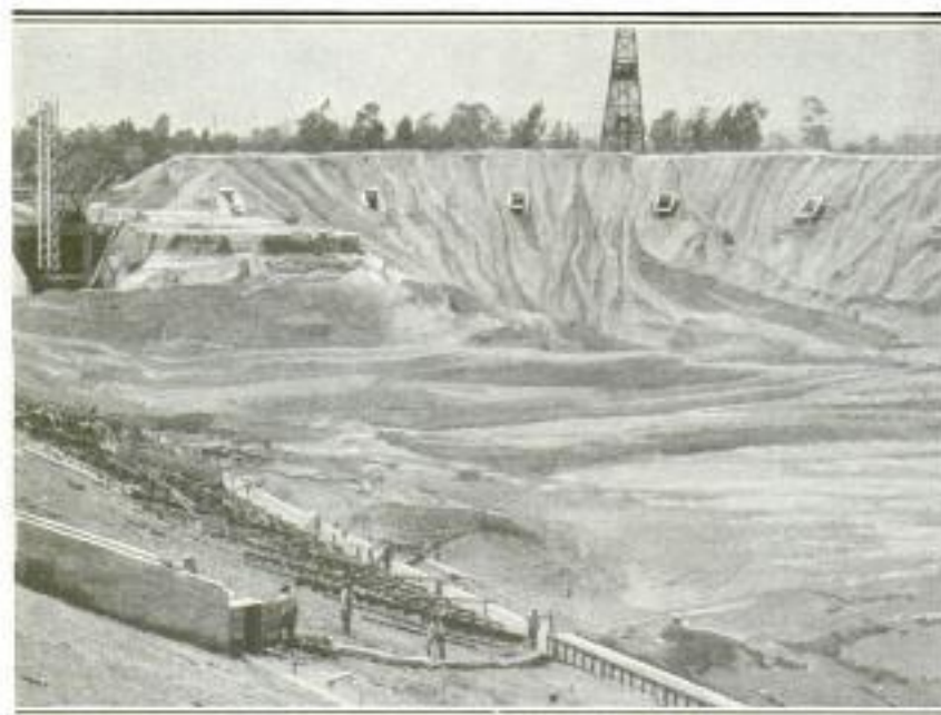
Bowl of Stadium during Construction: Note Rim, 79 Feet High, in Background, Compared with Derrick behind It; Also Forms for Concrete Construction in Left Foreground
