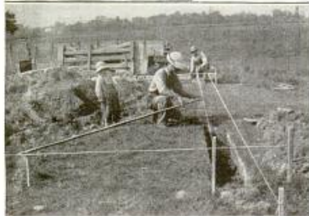
Laying Out Square Corners for Foundation Walls by Means of the 6, 8, and 10 Rule: This Is a Simple Method, and Quite Accurate
