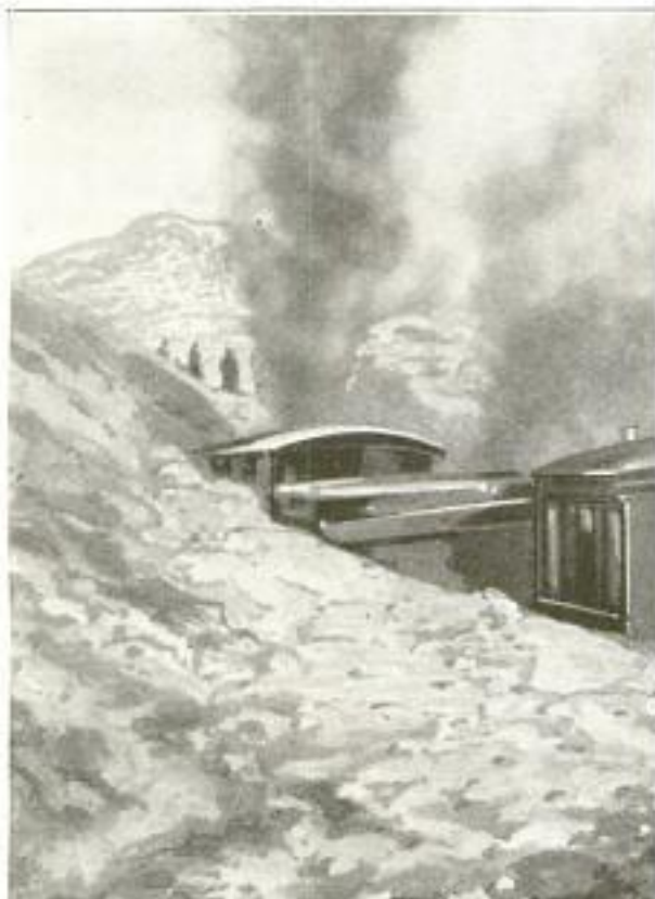
Clearing the Right of Way after an Alaskan Snow-storm: This View Shows the Hard Pulling a Snowplow must Do When the Drifts Are as Heavy as This One
