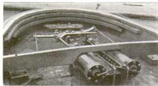
Connected with the Controller in the Wheelhouse, These Cylinders on Deck Actuate the Tiller of the Rudder
