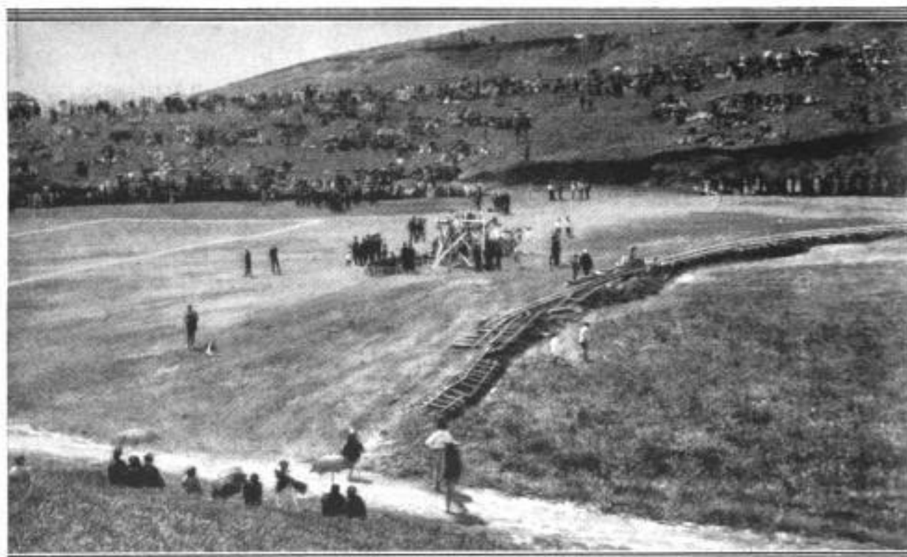
A View at the Site of a Stadium under Construction at Jalapa: This Is the First Stadium Built in Mexico and the Second in Latin America. It Has a Capacity of 30,000 and was Made by Filling a Swamp That Was a Breeding Place for Mosquitoes
