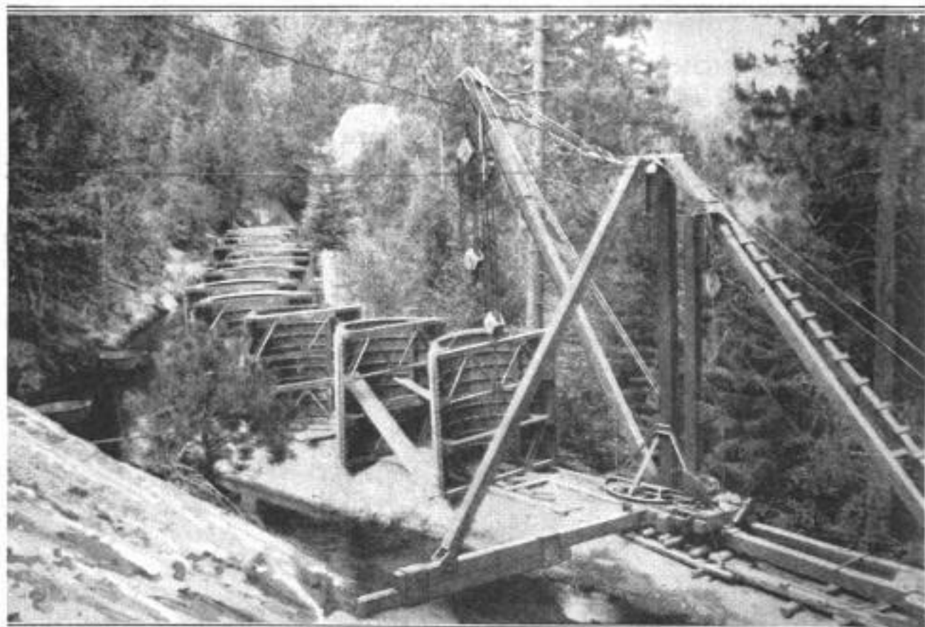
The Manner of Using a Derrick for Handling the Heavy Precast Sections of the Canal Lining, the Steel Forms and Bracing Facilitating Attachment to Derrick Tackle: Note Tub Containers in Left Background
