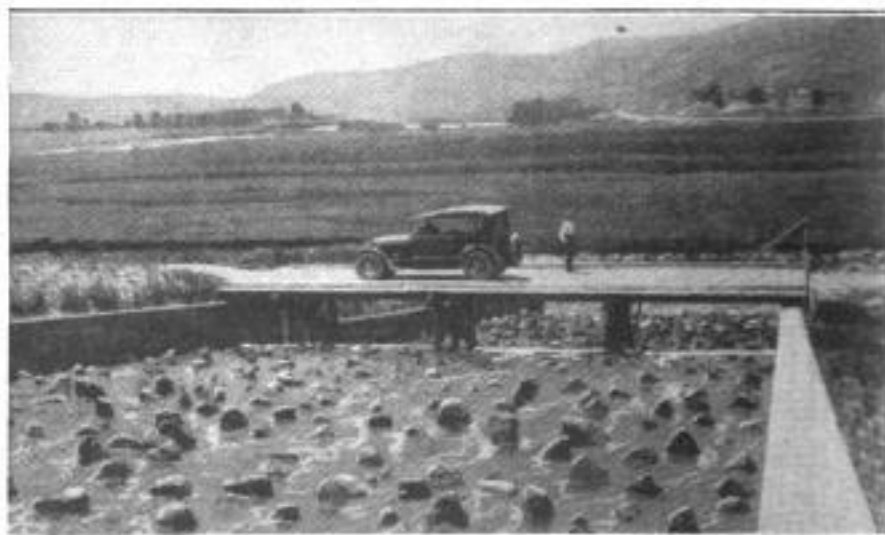
To Reduce the Speed of the Water in This Spillway, Emptying Directly into a Small River, Rocks have been Laid over the Floor, and a Slight Fall and Shallow Channel Built Close to the Junction
