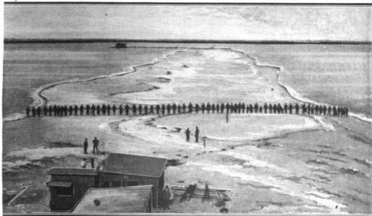
This Picture Shows the Immense Length and Width of the Causeway at the St. Petersburg Approach to the St. Petersburg-Tampa Bridge. Several Miles of This Causeway, to a Width of 400 Feet, have been Filled In
