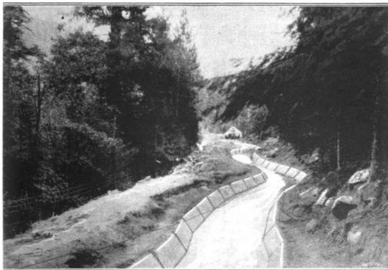
A Completed Section Lined with Concrete: The Reinforcing at the Ends of Each Precast Section is Tied In with That of the Abutting Section, Showing a Heavy Dark Line at Each Joint. Note the Adaptability of These Precast Sections for Following the Sinuous Course of the Canal. Before Facing Them with Concrete, the Curved Banks at This Point were Subjected to the Most Severe Erosion
