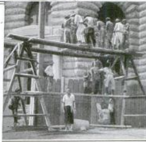
Driving Sheet Piling by Man Power for the Purpose of Holding the Slimy Mud in Place beneath the Foundation of the New Bank Building in Shanghai
