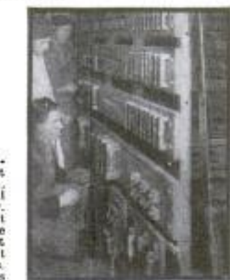
Rear view of one switch board. Students making repairs under personal direction of instructor Dillon.
