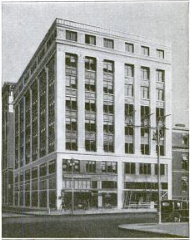
The Left Half of This Building is Completely Finished and Occupied by Tenants, While the Second Half is Still under Construction
