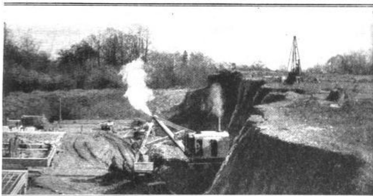
In Order to Provide Building Space for the Extension of a Chain of Apartment Buildings in Washington, District of Columbia, the Steam Shovel is being Used to Excavate Truckload after Truckload of Dirt from This Hill, Which is Used for Fill on Another Job
