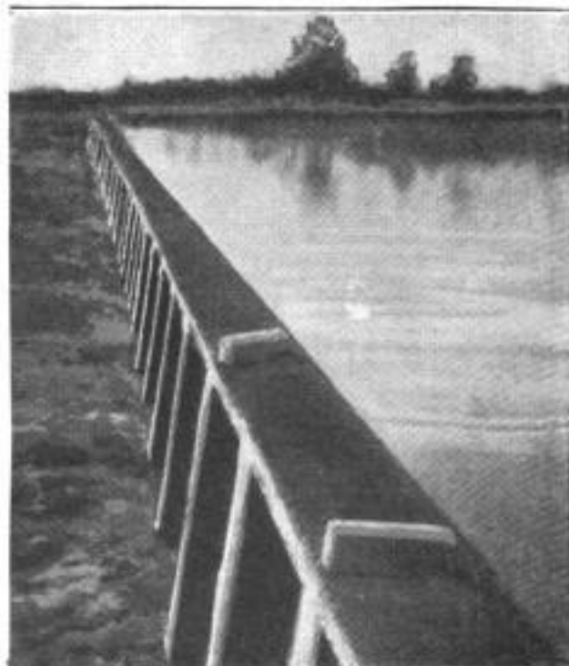
The Wedge-Shaped Wood Blocks, Seen along the Crest of This Dam, Stopped a Series of Mysterious Earthquakes in the Neighborhood
