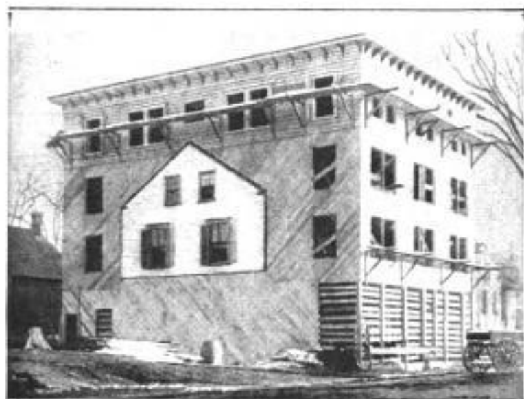
Four-Story Building Which was Erected around a Small Cottage, Showing One End of the Dwelling as Part of the Building Wall Before It was Entirely Finished
