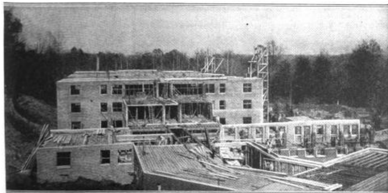
View during Construction of the Chain of Apartments That are being Extended as Fast as the Razing of the Hill Progresses: It is Estimated over a Million Truckloads of Dirt will be Moved
