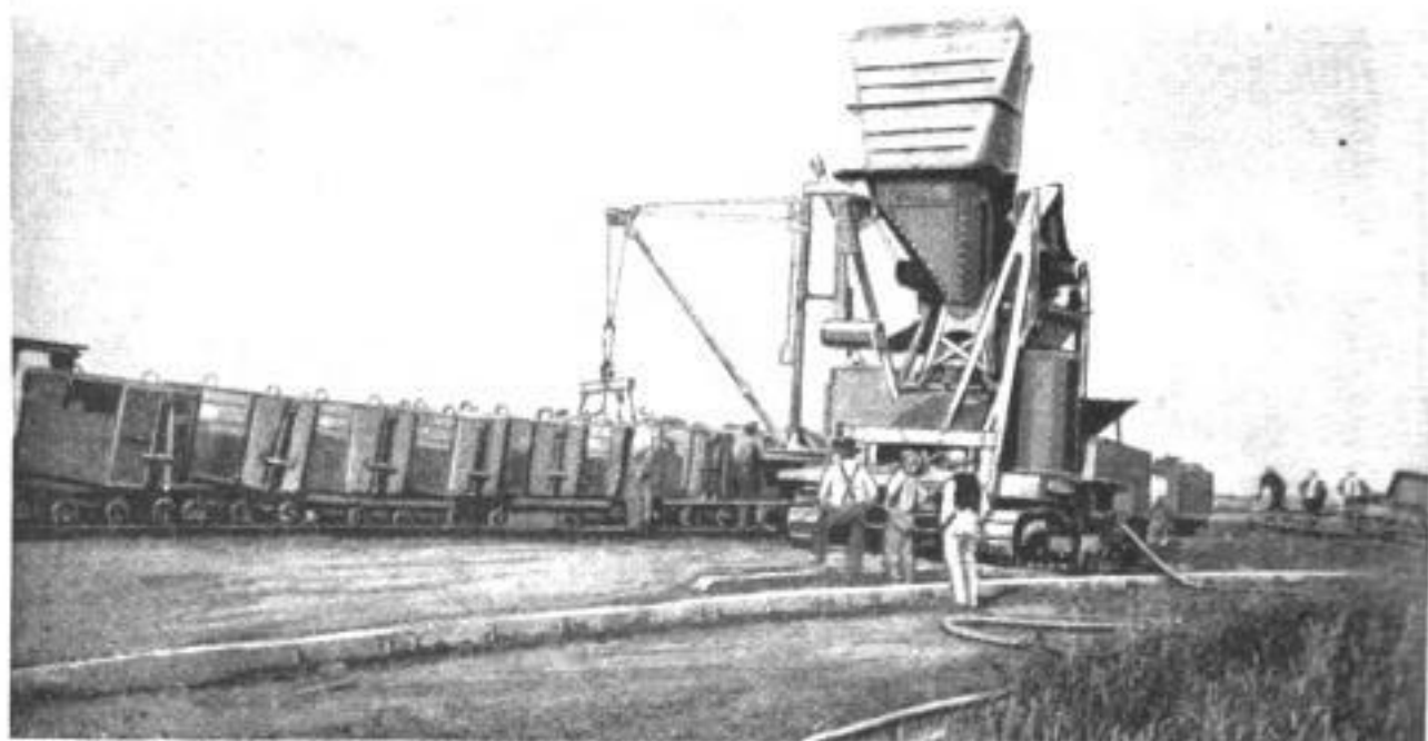
Another View of the World's Largest Paving Machine, Showing the Skip Elevated and Depositing Its Contents into the Mixing Drum: The Derrick is Seen Putting the Empty Car Back on Its Truck, Which Forms Part of the Long String of Cars That Are Necessary for the Operation of the Equipment
