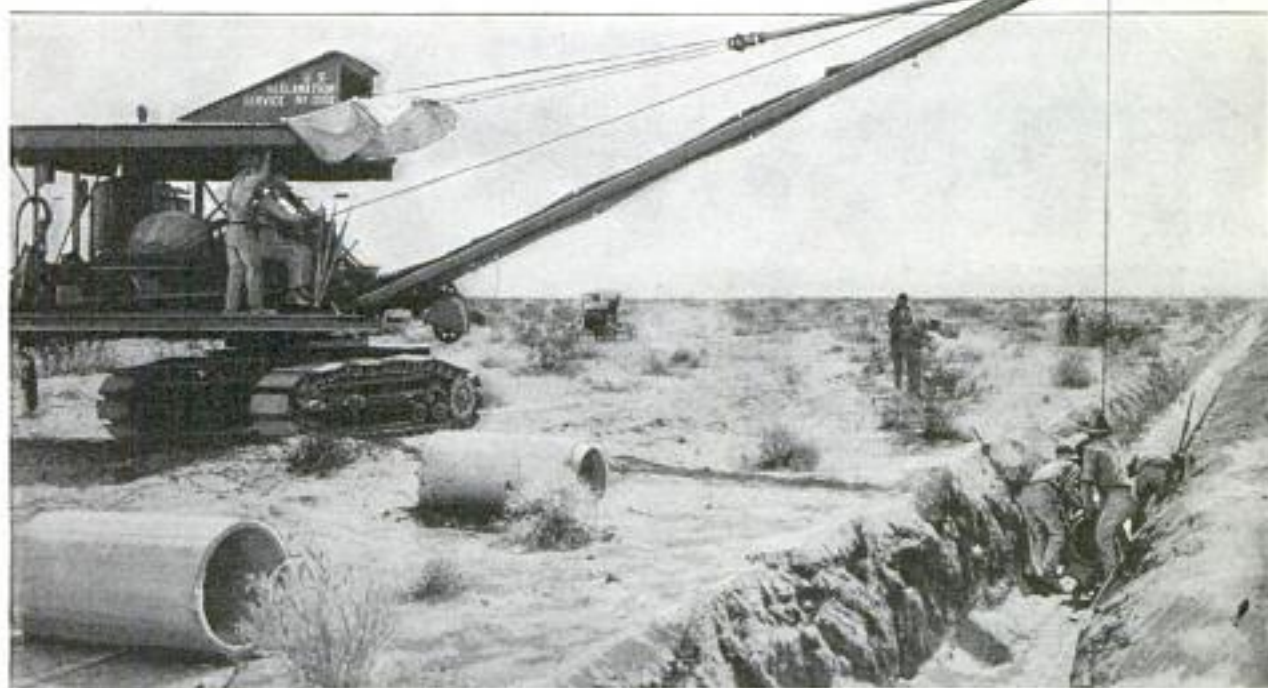
Laying 18-Inch Concrete Pipe with a Dragline Excavator on the Mesa of the Yuma Land Project: In This Manner One-Quarter of a Mile of Pipe was Laid and the Joints Sealed Every Day
