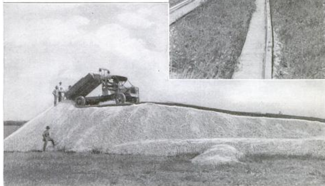
Above: View Showing the Runways Which are Built in Interchangeable Units, 10 Feet Long, and Laid Down for the Truck Used in Building the Stock Pile. Below: Side View of the Stock Pile, Showing Truck Dumping a Load of Crushed Stone
