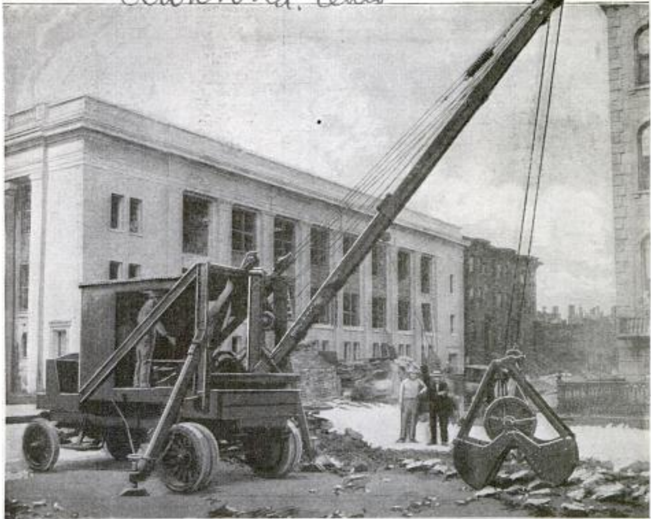
This Locomotive-Type Crane can be Mounted on Any Five-Ton Motor Truck Measuring at Least Nine Feet from the Back of the Driver's Seat to the Center of the Rear Axle. Nearly Worn-Out Trucks can be Used for This Service
