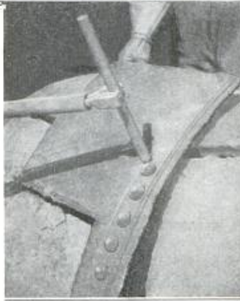
The Arc Cutting Tool being Used in Cutting Out Rivets by Melting Off Their Heads
