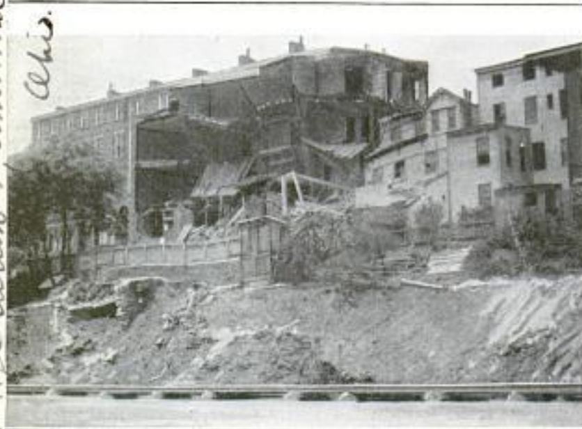
Apartment House Which was Dynamited by Wrecking Crews, Showing Part of the Structure Demolished
