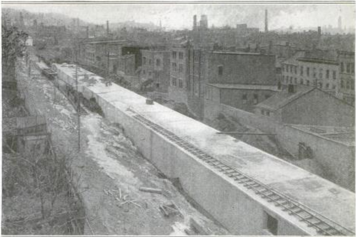
View of One of Cincinnati's Subway Tunnels, Showing the Completed Concrete Work before Backfilling: Note the Small Track on the Roof of the Tunnel, Which Carried the Concrete Cars from the Mixer to the Forms
