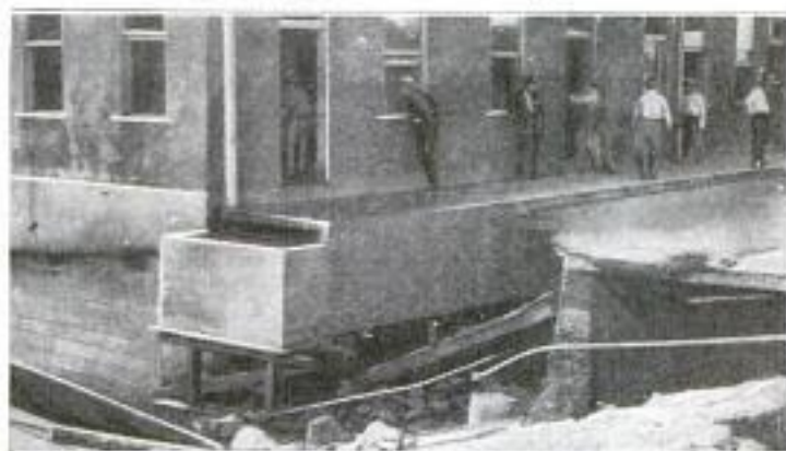
Flood Damage Done to Offices of Custom, Immigration, and Health Departments Located at American End of International Bridge across the Rio Grande
