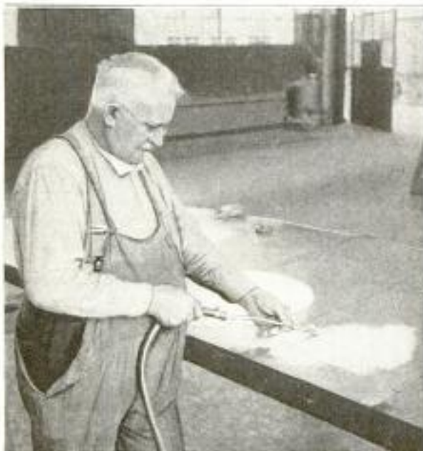
Blistered-Paint Remover Which is Operated by Means of Compressed Air, Showing the Special Scraper Attached to the Air Hose
