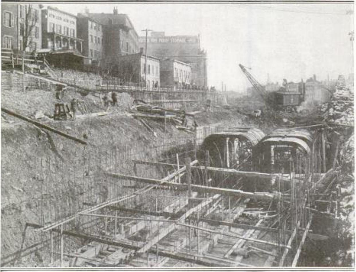
Above: Vertical Reinforcing Bars That Form Part of the Side Walls of the New Cincinnati Subway Tunnels. Below: Excavation for Subway, Showing Bottom Concrete in Place, and Side Wall, as Well as Some of the Arched Forms
