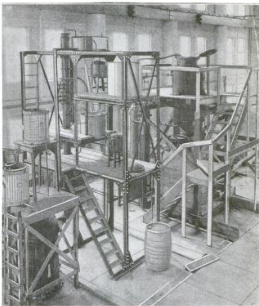
Stills and Condensers of the Development Unit Used by the Bureau of Chemistry, Department of Agriculture, in the Extraction of By-Products from Corncobs
