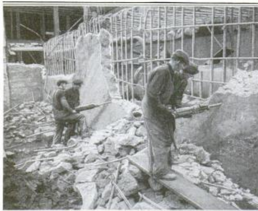
Part of a Reinforced-Concrete Wall being Destroyed by Pneumatic Hammers, Each Operated by Two Men to Make the Work Speedy: The Reinforcing Rods Still Standing were Broken Up Later with Cutting Tools
