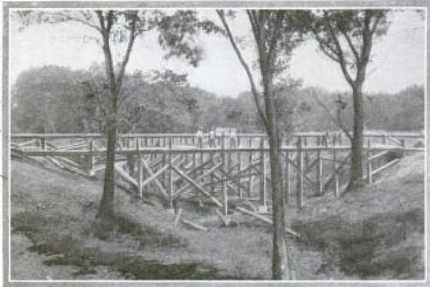
Bridging a Ravine Where a Concrete Structure will Carry the Speedway Tracks for a Distance of 125 Feet and Form One of the Tunnels Leading to the Infield
