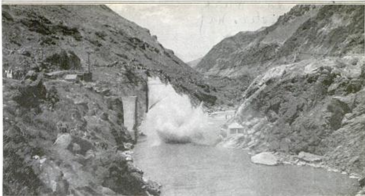
One of the Columns is Seen Here Just as It Falls into the River, being Broken at the Notched Point by a Charge of Dynamite. The Standing Column Shows Where the Notch was Cut
