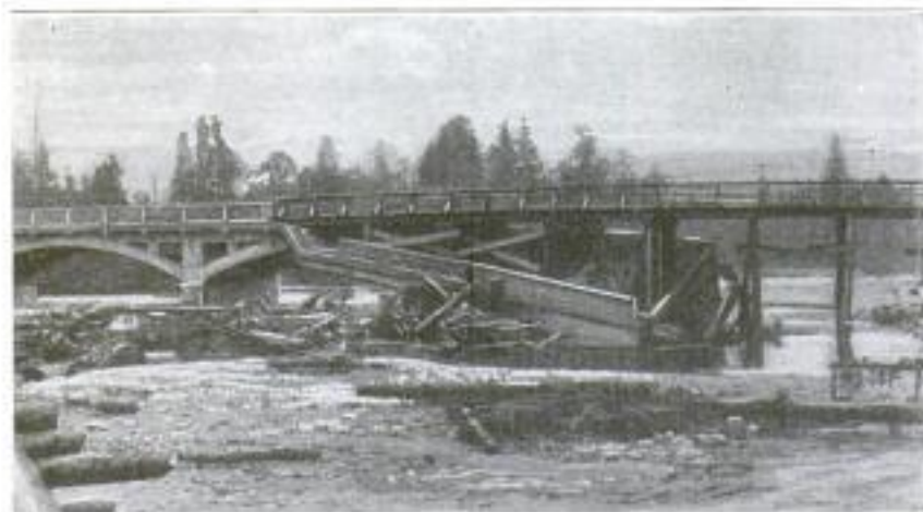
Wreck of Highway Bridge, above the Railway Bridge, Caused by the River during One of Its Flood Periods
