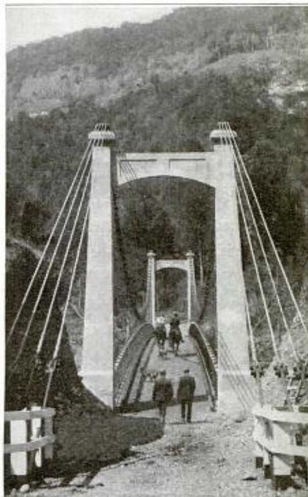
Another View of the Bridge: The Towers Are 25 Feet High, the Bridge Deck Is of Reinforced Concrete and 12 Feet Wide
