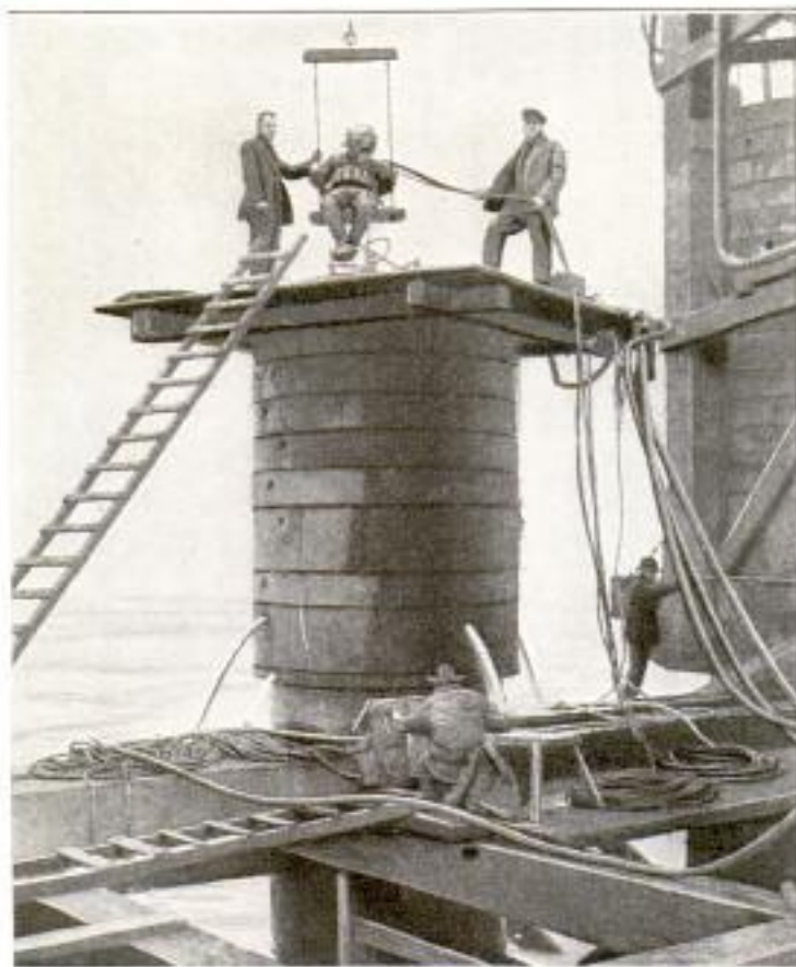
Diver Returning from Inspection Trip to Bottom of Huge Concrete Pile, Nearly 100 Feet below Surface of Harbor: The Water Pouring Out of the Holes in the Heavy Cast-Iron Rings, Comes from Hydraulic Jets Employed to Aid in Sinking the Pile
