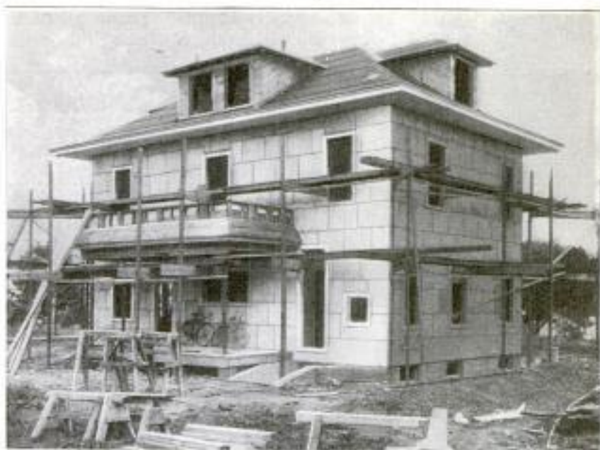
Dwelling, with Siding Made of the New-Process Concrete: The Outside Face of the Slabs will be Covered with Stucco, Their Air-Cell Structure Making Them Good Heat and Sound Insulators
