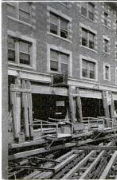
Upper Right: General View of Hotel Building in the Process of being Moved through City Street. Lower Left: Close-Up, Which Shows Timbering Necessary to Support Upper Floors While Moving, Also Timbers and Rails along Which the Building was Pulled
