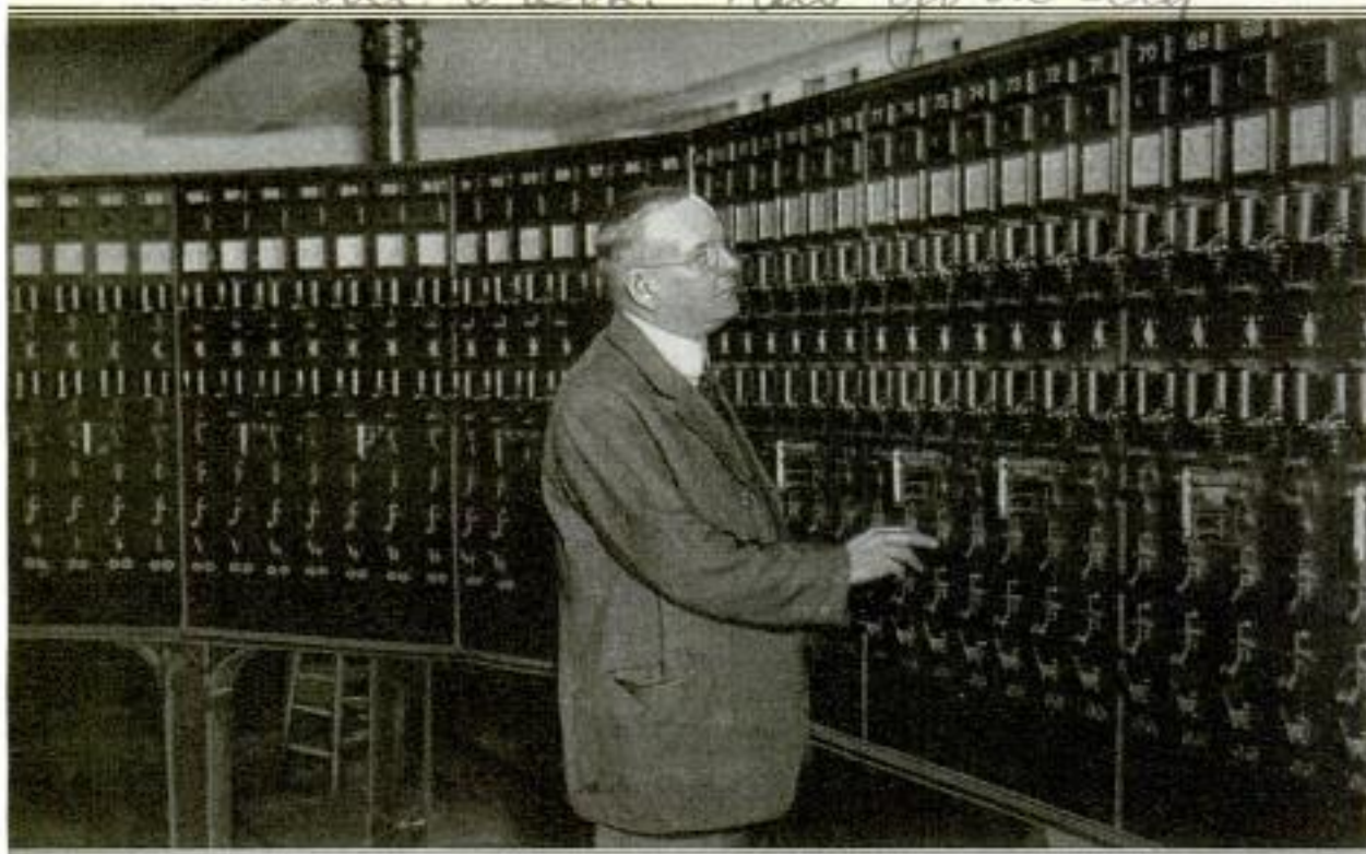
The Relay Receiving Board of the New York Fire-Alarm System, Which Distributes the Alarm to the Proper Stations, with Little Loss of Time, and Thus Assists in Speeding Up the Answering of Calls
