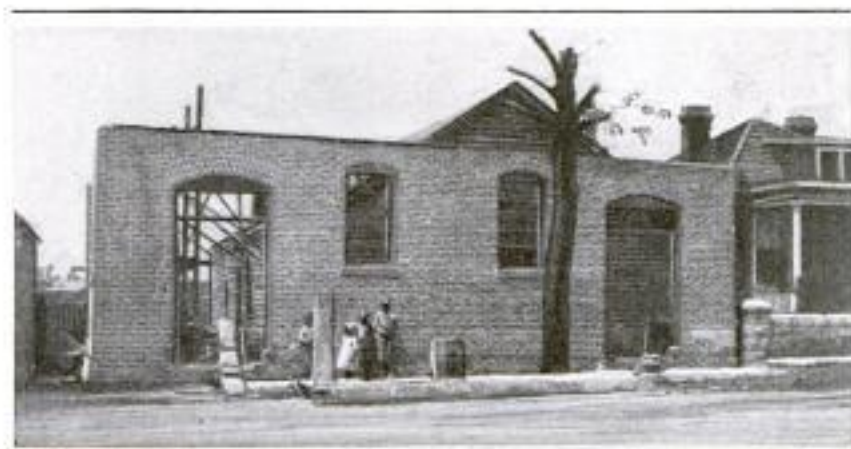
The New Brick Church of a Negro Congregation in Lexington, Kentucky, under Construction around the Old Wooden House of Worship
