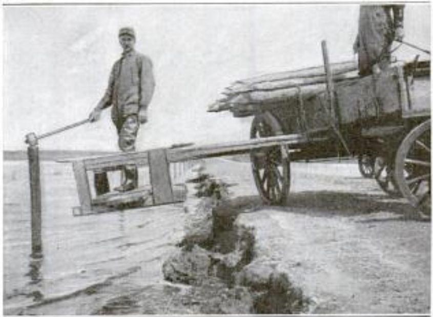
A County-Road Commissioner of South Dakota Standing on the Makeshift Platform Which He Built to Enable Him to Drive Posts in the Water in the same wagon from which the platform was built.
