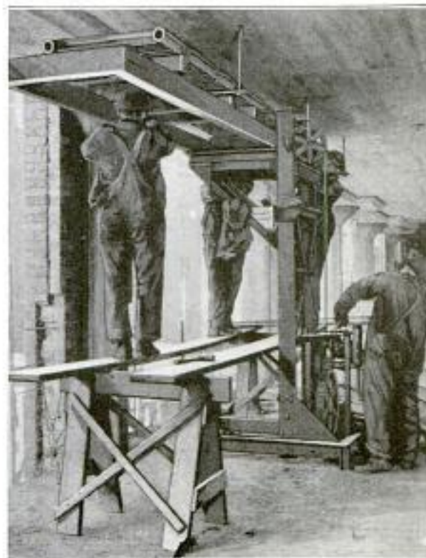
An Unusual Job for the Box-Stacking Machine: It is Here Used by a Gang of Millwrights to Hoist Fittings to the Ceiling of a Shop
