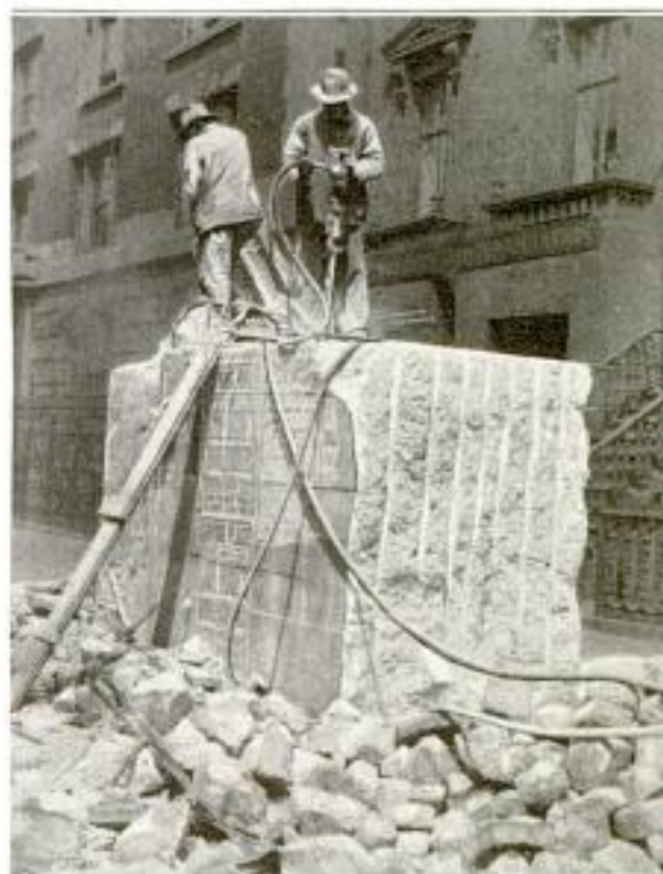
Above is Shown Men at Work with Air Drills, Making Holes in a Large Concrete Anchorage, Preparatory to Breaking It Up with Wedge and Sledge Hammer
