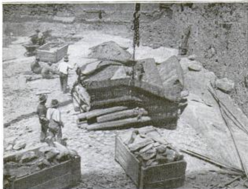
Raising the Wire-Cable Matting after a Blast: Under It Is Another Mat of Two-Inch Rope, and at the Sides Heavy Log Buffers
