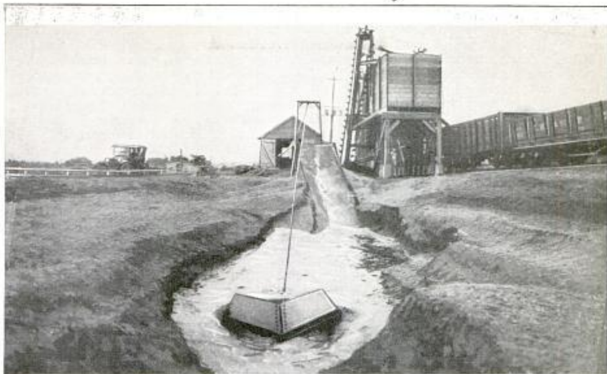
This Power-Driven Scraper Scoops the Gravel from the Bank and Delivers It to the Elevator Which Carries It to the Storage Bin, and from There It Goes to the Waiting Railroad Cars
