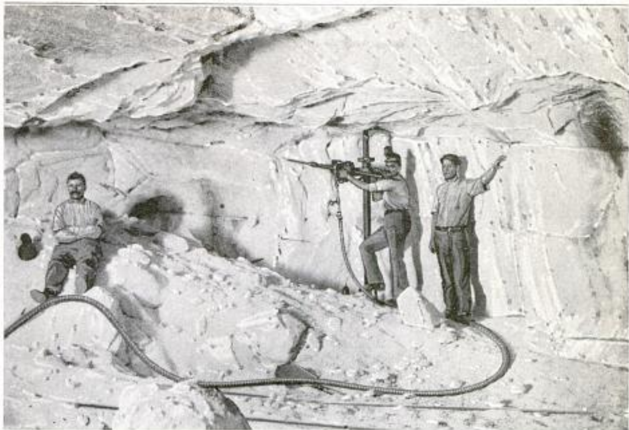
Where the Salt has been Recently Blasted, the Surface Is a Glittering, Silver-White Mass. At This Point, a Drill Operated by Compressed Air is being Used to Make the Holes That will Receive the Charges of Dynamite for Breaking Down the Salt
