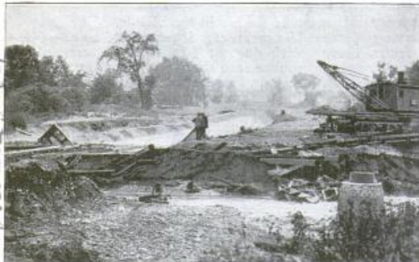
Part of the Wreckage Caused by the First Cloudburst That Syracuse, New York, Ever Experienced and Which was Followed in a Week by a Second
