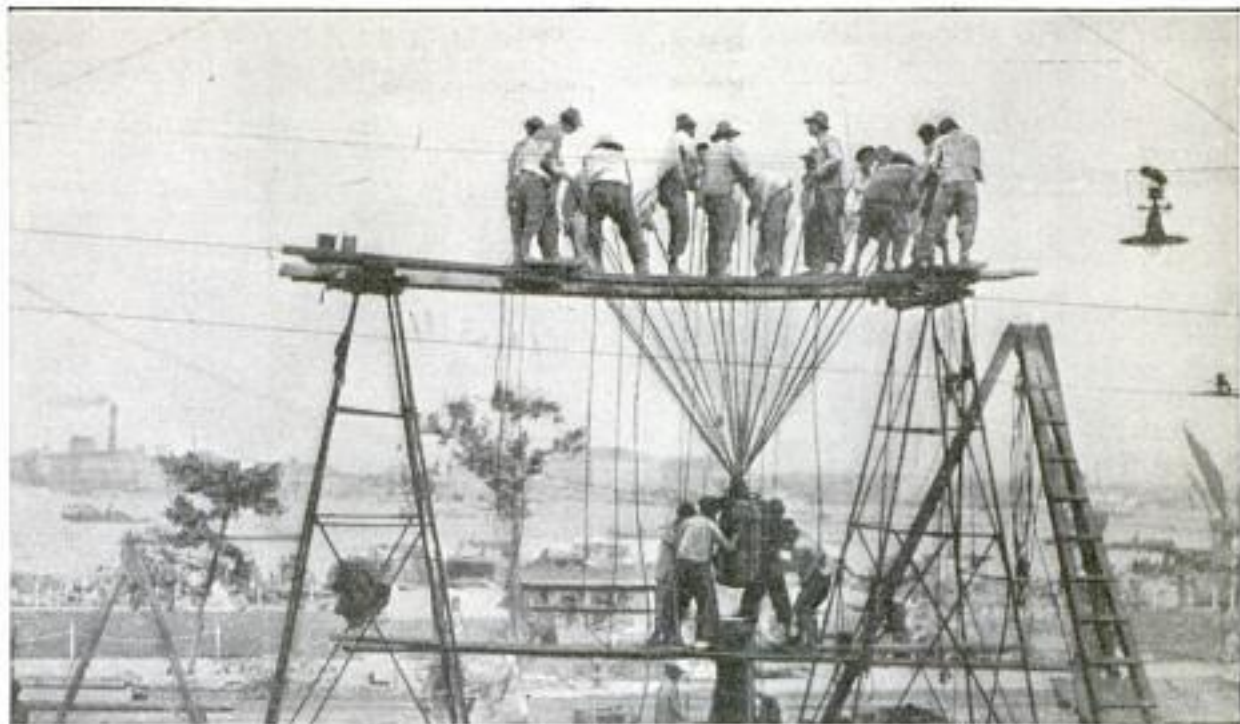
These Coolies are Working on Shanghai's First Sewer System, Singing, as They Work, the Ancient Pile-Driver Chant under the Leadership of a Special Overseer
