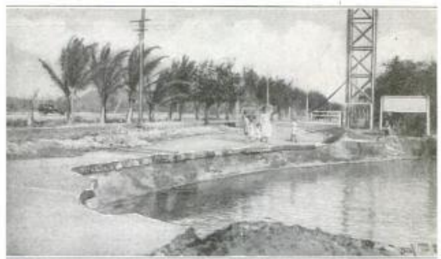
Palm-Lined Boulevard in Honolulu as It Appeared After the Large Dredger had Partially Completed the Task of Cutting through the Pavement
