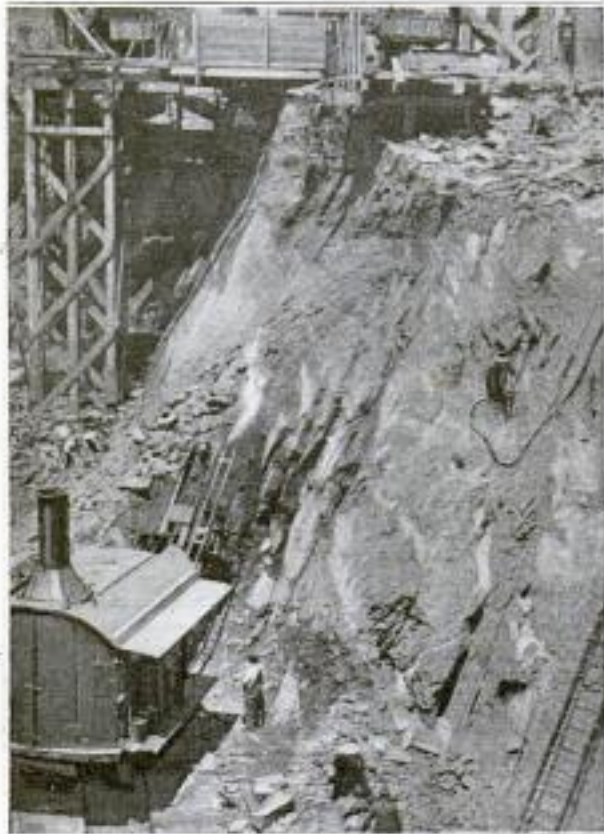
New York's Deepest Solid-Rock Building Excavation: It Goes to a Depth of 42 Feet. An Addition to a Large Store will be Erected Here
