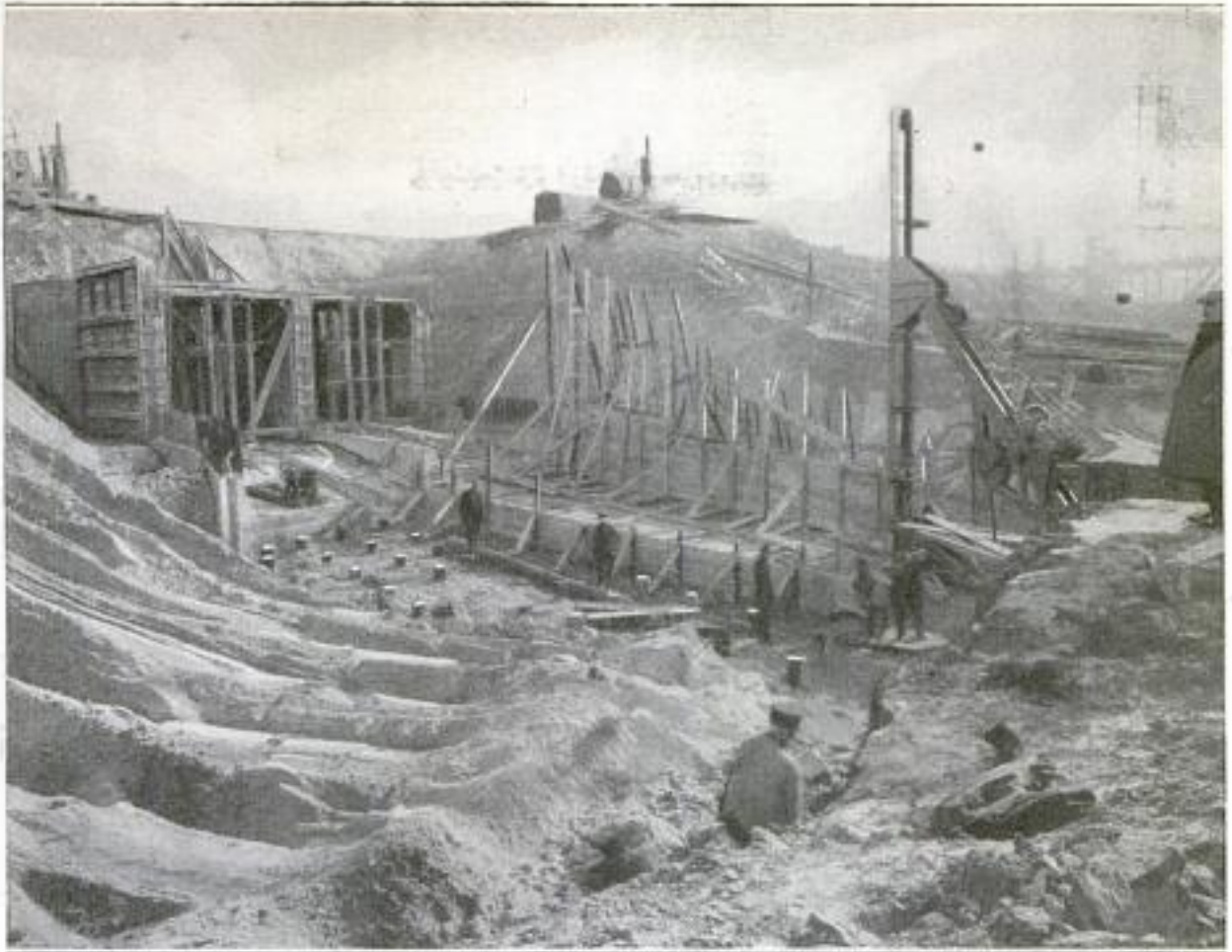
This Shows Excavation and Construction Work Progressing on the Outfall Portion of the Main Sewer, Where It Empties into the Kansas River, and Gives Some Idea of Its Immense Size
