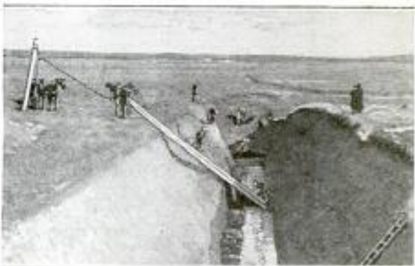
Skid Arrangement Used to Remove Excavated Material from an Open Sewer Trench: The Soil was Wheeled to the Bottom of the Runway and Dumped into a Drag Scraper, Which was Drawn to the Surface by a Team of Horses
