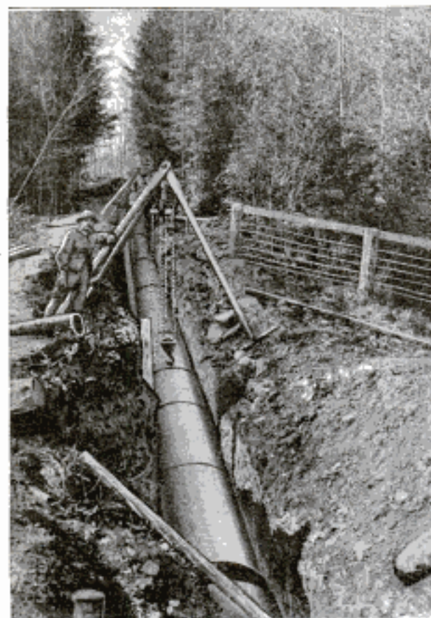
This Steel Overflow Pipe, Welded after being Placed in Position, was Buried in the Ground to Reduce the Effects of Temperature Changes
