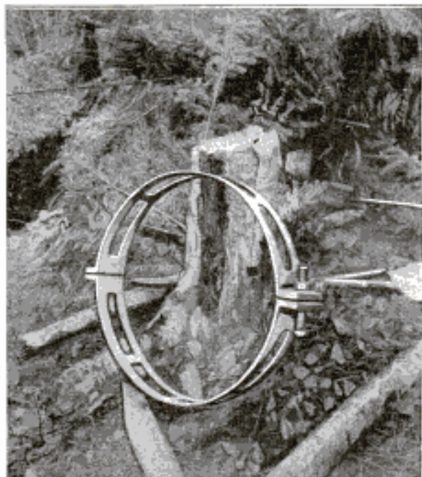
The 20-Foot Lengths of Pipe were Drawn Together and Securely Held by This Clamp While the Welding was being Done with Gas Torches
