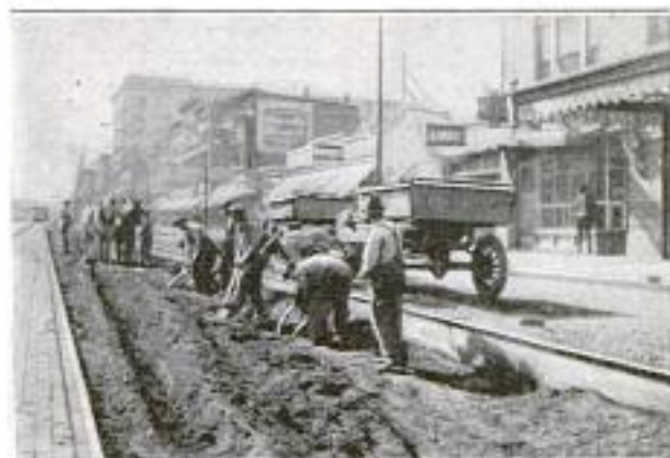
This Shows How the Header Curbs Act as Retaining Walls and Boundary Marks When Maintenance Work is being Performed on the Street-Car Tracks
