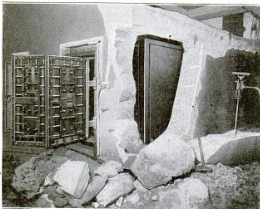
When Removing the Protecting Concrete from This Steel Vault, Holes were Drilled with a Compressed-Air Drill, and the Concrete Broken Away by Driving Steel Pins into the Holes
