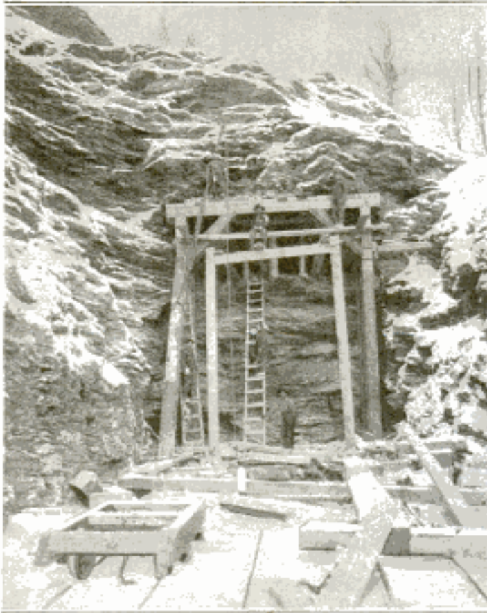
This Shows Work Progressing on One of the Tunnels along the Route. In Some Cases It was Deemed Advisable to Drive Tunnels Rather than to Make Deep Open Cuts through the Rock. The Formation at This Point Is Hard Slate
