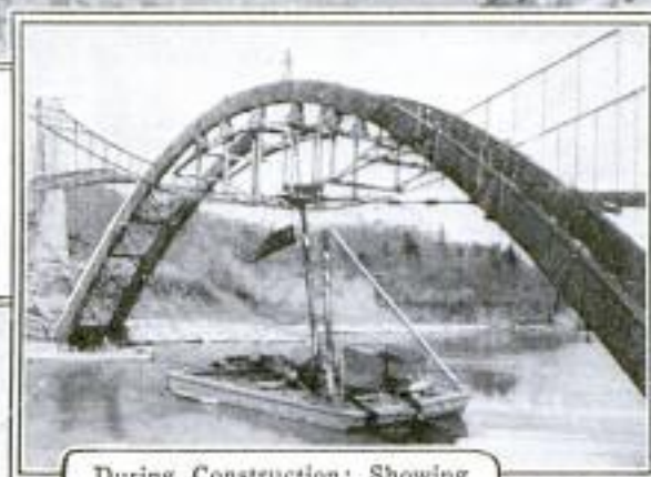
During Construction: Showing How the Cables of the Old Suspension Bridge were Used in Transporting Material for the New Structure
