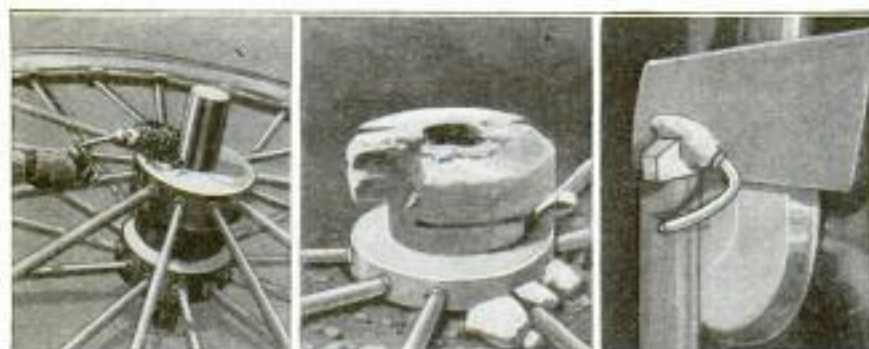
Left: A Sheave Wheel from the Headframe of a Coal Tipple, Removed without Injury to the Shaft. Center: The Effect of Two Charges of Explosive on the Sheave Hub. Right: Blasting Out a Tight Key
