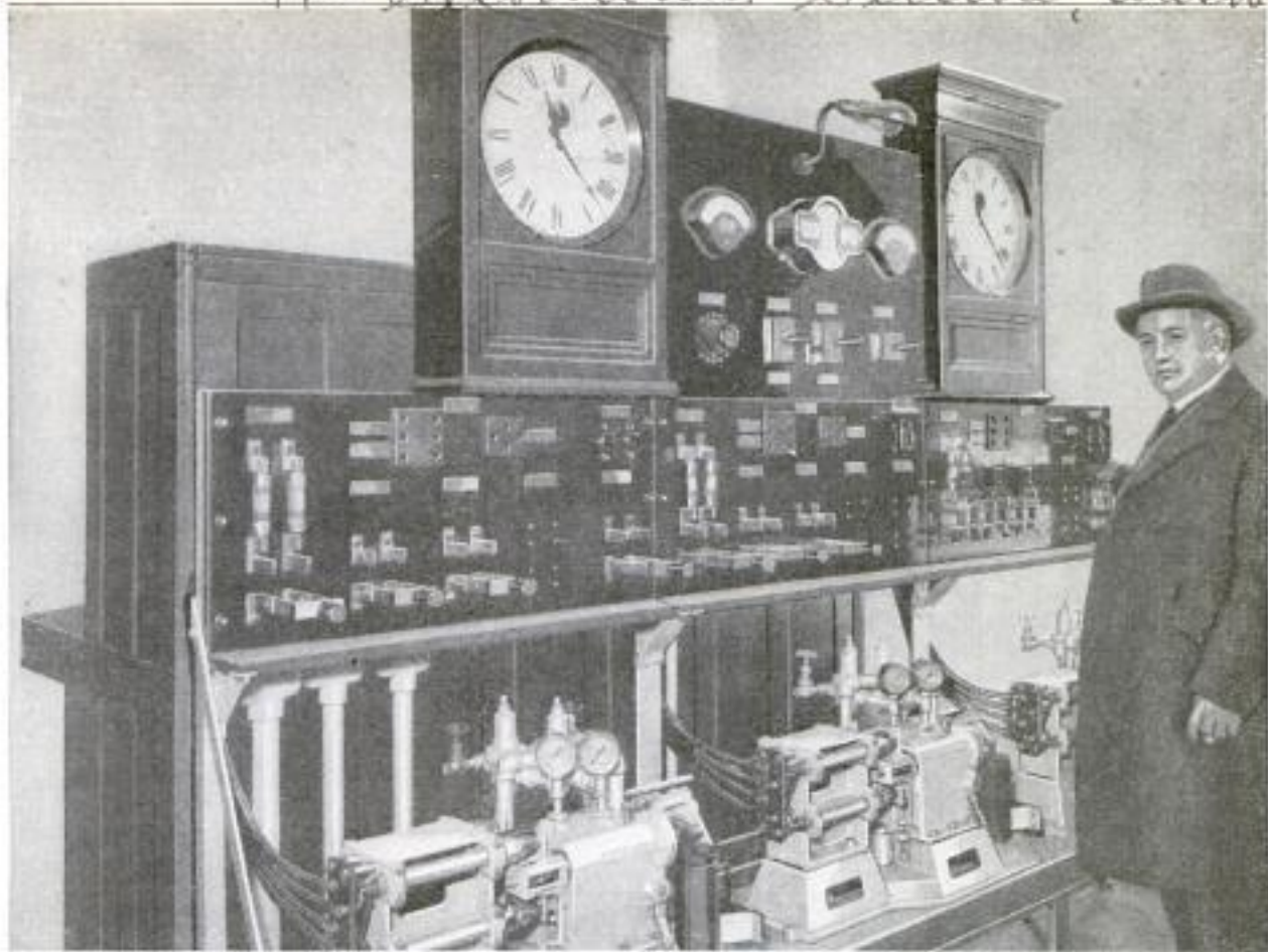
Electrical Equipment Which is Installed at the Central Office to Operate the Measured Telephone-Service System: The Two Duplicate Time Clocks are Seen Above and the Pole-Changing Switches Below, Together with Meters, Knife Switches, Fuses, and Other Necessary Apparatus
