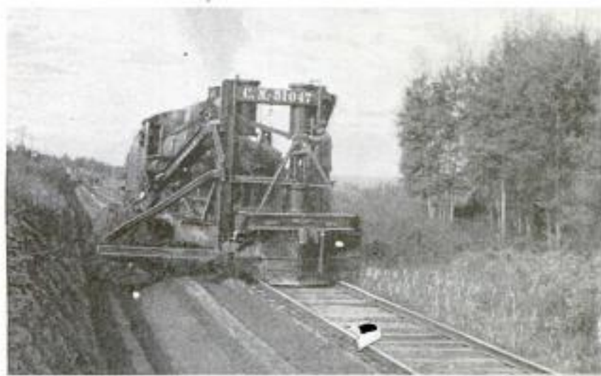
Last Run of Ditcher being Made with Steel Template on the Bottom of the Wing to Finish the Roadbed Shoulder, the Ditch, and the Side Slope to Standard Form
