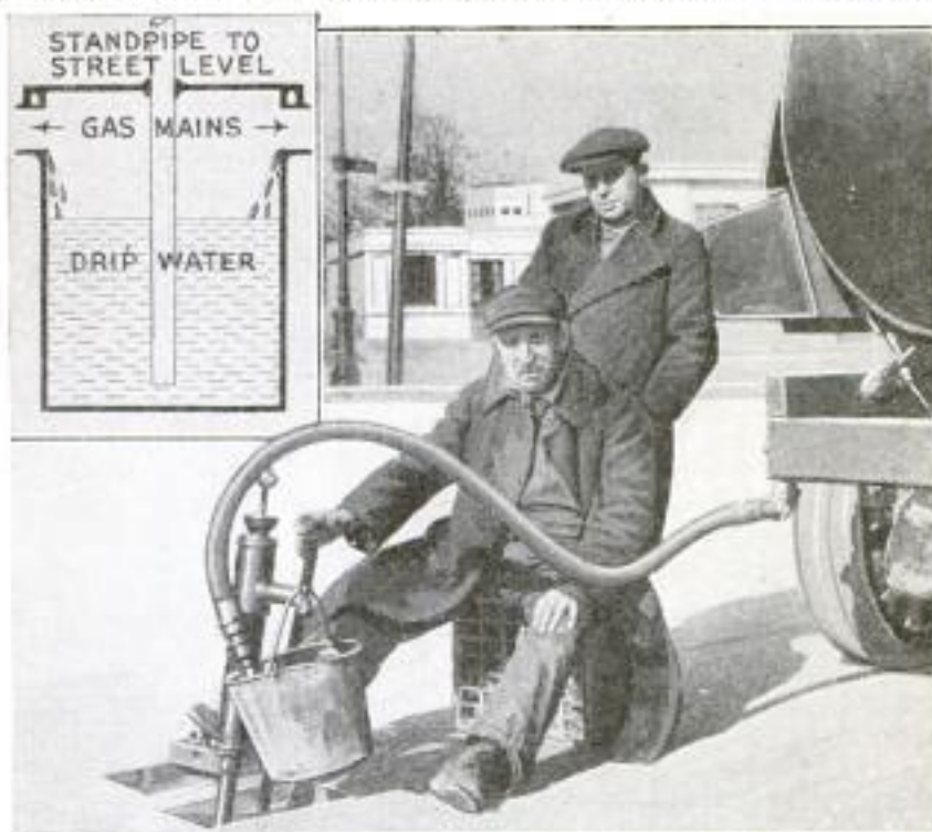
Hand-Pumping the Drip Water from One of the Drip Wells into a Bucket, from Which the Water is Pumped by a Motor into a Tank Truck: The Insert Shows a Cross Section of the Drip Well
