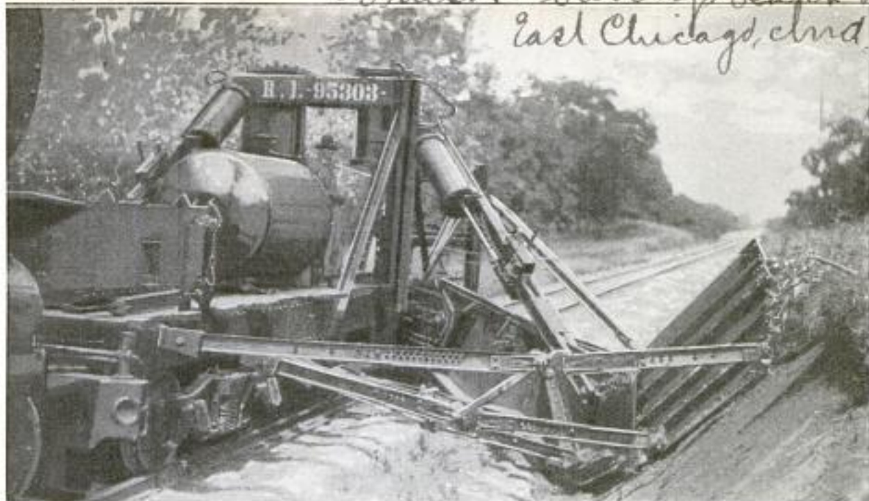
Wing-Type Ditcher at Work on a Railroad: The Wing or Scraper Attached to the Heavy Car, Which is Moved by a Locomotive on the Track, is Adjusted to Give the Desired Section to the Ditch at the Side of the Roadbed. The Wing Cuts the Soil and Shoves It Ahead
