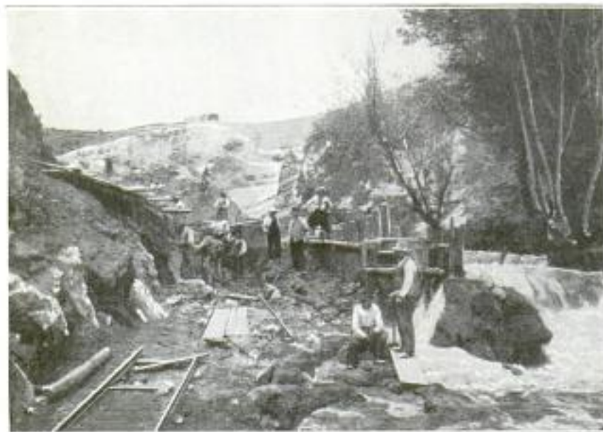
Construction Work Progressing on the Hydroelectric Power Flume Which will Carry Water from a Well That is Traditionally Believed to have Sprung from a Footprint of Abraham
