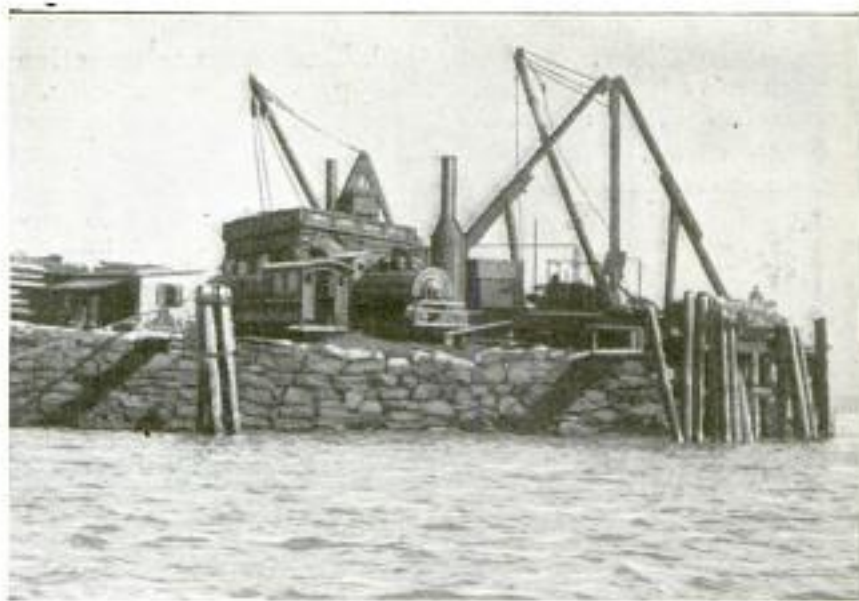
Landing Place and Equipment: Watchman at Right of Derrick Reports Presence of Anyone Attempting to Land on Island from Boats
