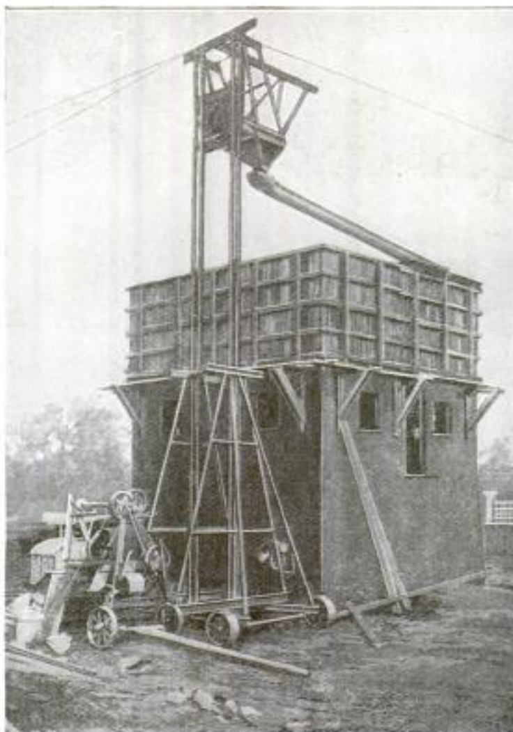
Monolithic-Concrete House under Construction: Wooden Forms for Upper Story Are in Place, and Concrete is being Poured from the Telescoping Portable Tower with Its Funnel-Shaped Outlet, Which is Raised to Its Full Height
