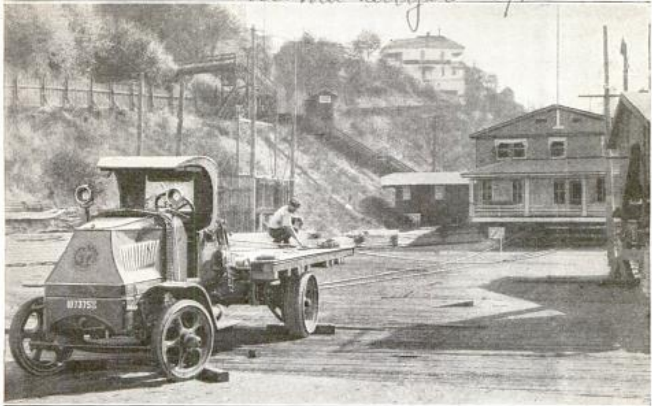
Motor Truck Moving a 250-Ton Office Building, in Portland, Oregon: The Truck was Blocked, and a Winch, Driven by Its Engine and Mounted Just behind the Seat of the Machine, was Used to Move the Heavy Structure a Little at a Time
