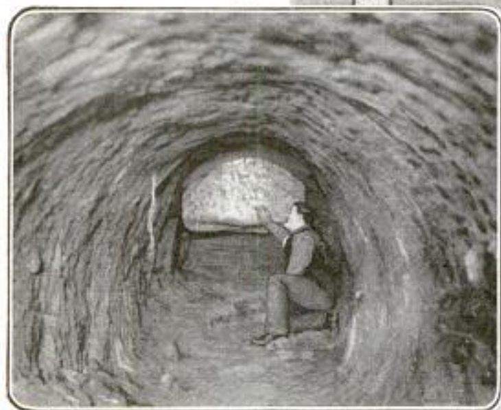
End of Tunnel to Unsupported Base of Foundation Pier: Bottom of Pier, at the Man's Hand, had been Pushed Down from Top of Tunnel by Load of 260 Tons.
