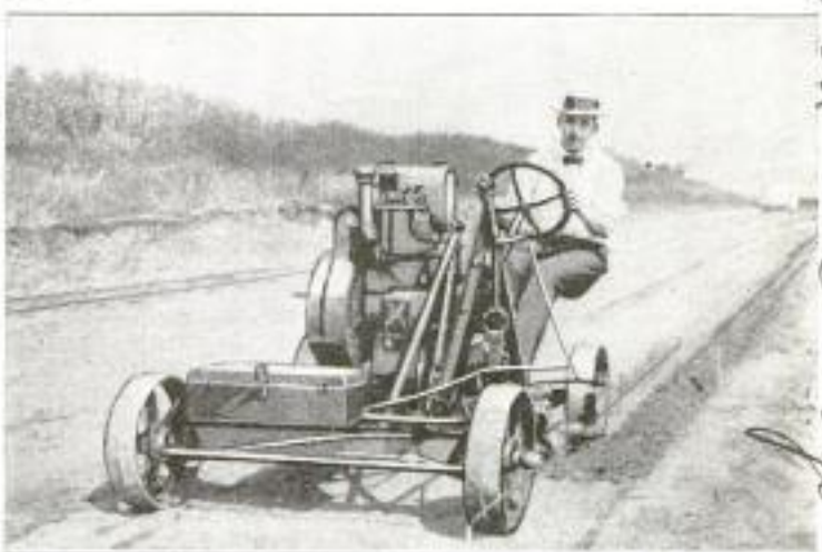
Steered along a Chalk Line, This Machine Cuts an Eight-Inch Trench True to Grade and Leaves the Bottom Solid
