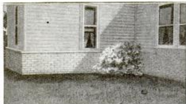
Building a Low Cement Wall around a House to Improve Its Appearance: The Owner has Found That the Floors of the Dwelling Are Now Much Warmer in Winter Than Formerly
