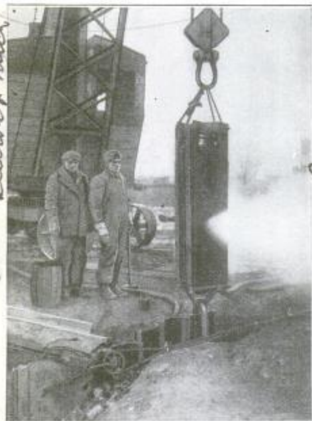
Steam Hammer, Slung from Derrick in Upside-Down Position, Drives Frozen-In Piling Upward by Means of Cable Slung over Hammer and Connected to Piling
