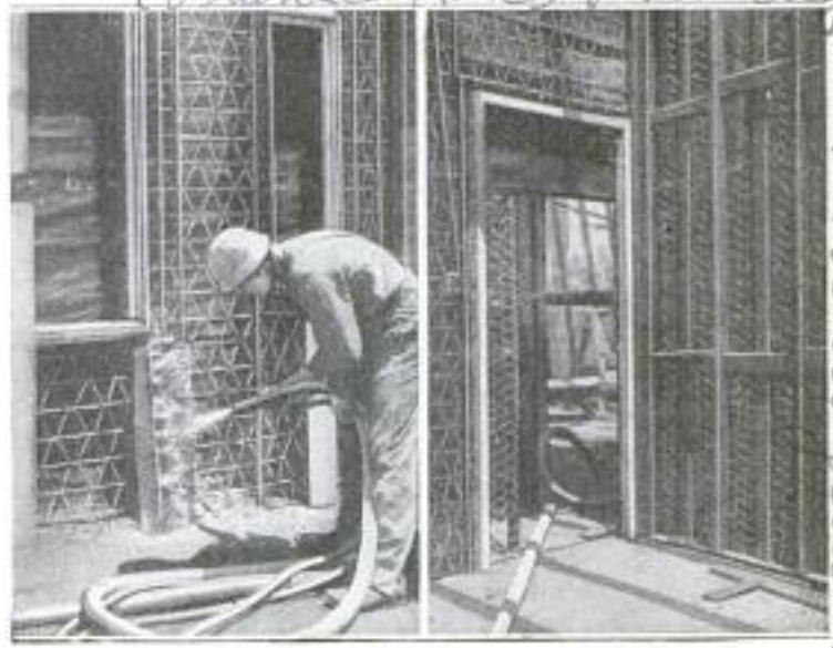
Interior of the Bungalow, Showing the Method of Shooting the Concrete around the Door and Window Frames
