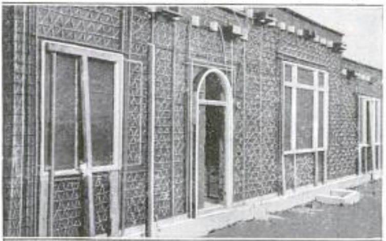
Exterior of the Bungalow, Showing One of the Outer Walls before Shooting the Concrete Mixture against the Framework
