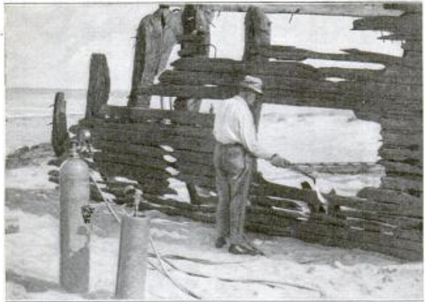
Means Employed by a Motion-Picture Company to Counterfeit the Weather-Beaten Hulk of a Wrecked Ship: An Acetylene-Torch Outfit was Used to Burn Away and Char the New Lumber
