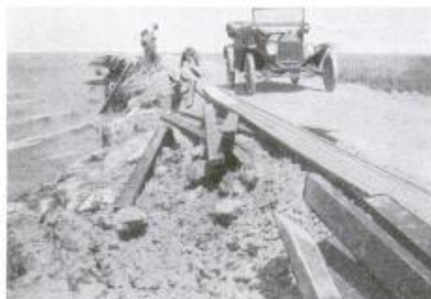
Timbering the Levee to Prevent It from being Washed Away by the Waves: The Water Here Stood 17 Feet Deep against the Levee
