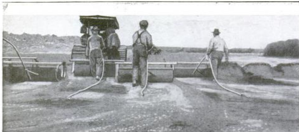
Hauling Five Four-Horse Scrapers by Means of One 45-Horsepower Tractor to Build a Levee to Protect Growing Grain from Threatened Floods: This Battery of Scrapers Makes It Possible to Build a Levee Three Feet High and One Mile Long in 12 Hours
