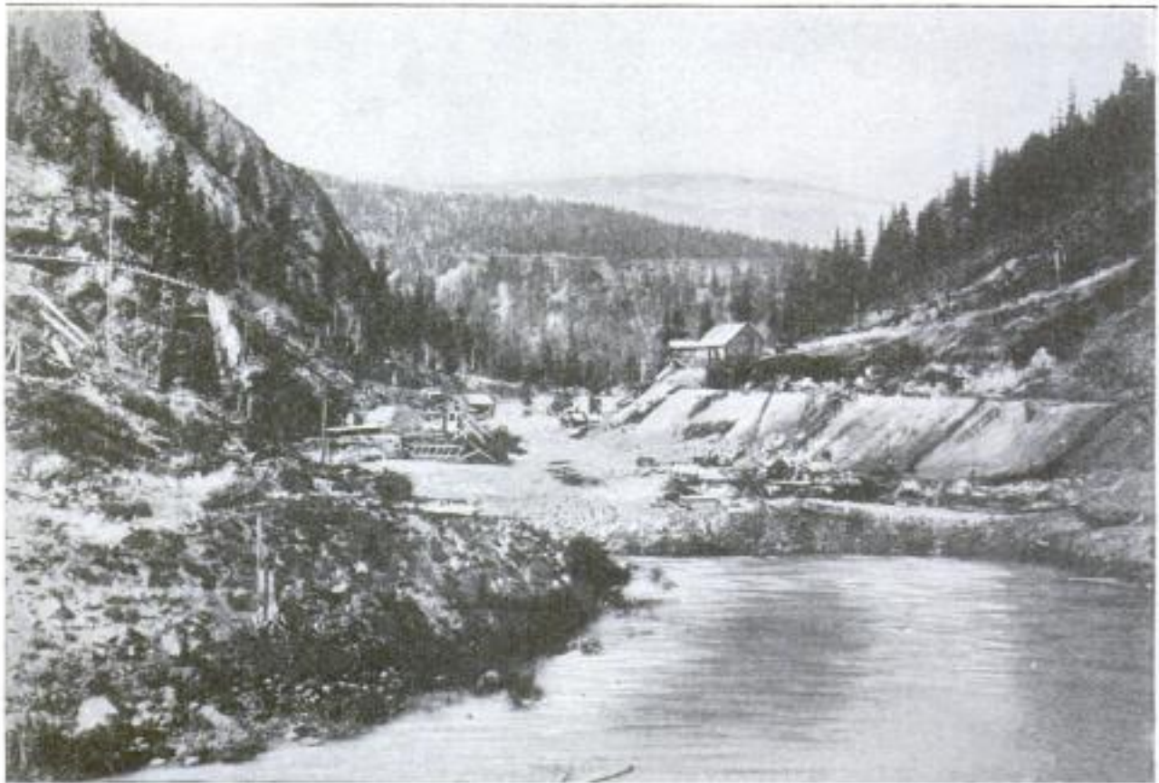
Site of the Tieton Dam, Which will Rise to a Height of 230 Feet, Being One of the Highest Earth Dams in the United States: A Corewall of Concrete will Extend through the Center of the Dam for the Full Width of the Cañon
