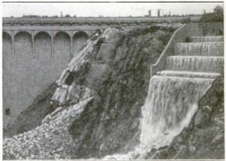
The Spillway Acts Only as an Emergency Overflow in Case of a Sudden Rise of Water in the Storage Reservoir
