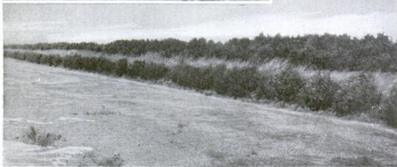
Above: Digging Machine Working on Levee to Protect the Enormous Wheat Field, Seen at Left, from Danger of Floods. Below: Looking from Lake toward a Section of the Levee That Bounds It. Two Rows of Willows on Lake Side are Planted to Protect the Soil from Waves
