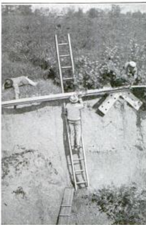
Carrying a 12-Foot Aid Post up a 20-Foot Bank, on Top of Which It is to be Erected
