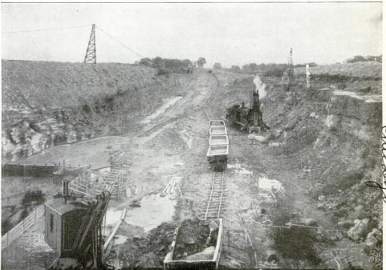
Excavations in Connection with Initial Work on the First Lock, near Marseilles, La Salle County, for the Illinois Waterway Improvement That will Make It Navigable for Large Steamers from Chicago to the Gulf of Mexico: The Lock will Be Parallel with the Illinois River, Which Is in the Background near the High Tower
