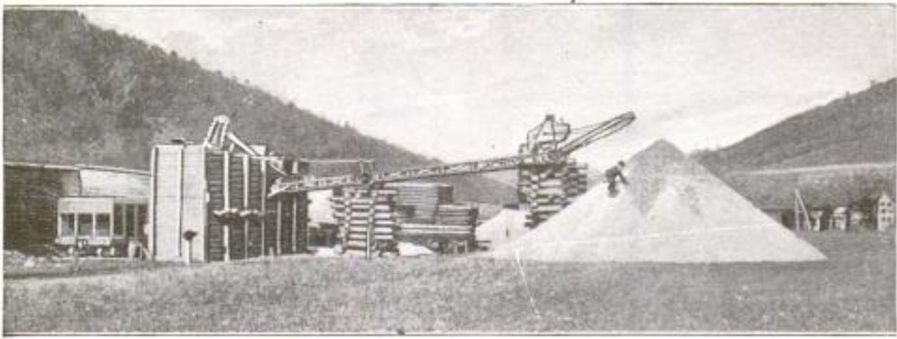
Conveyor for Unloading and Storing Stone for Future Use in Highway-Construction Work: The Conveyor is Supported on Cribbing Made of Railroad Ties Which are Added To as the Height of the Stone Pile Increases. It is Claimed That 50 Tons of Stone an Hour can be Piled in This Manner
