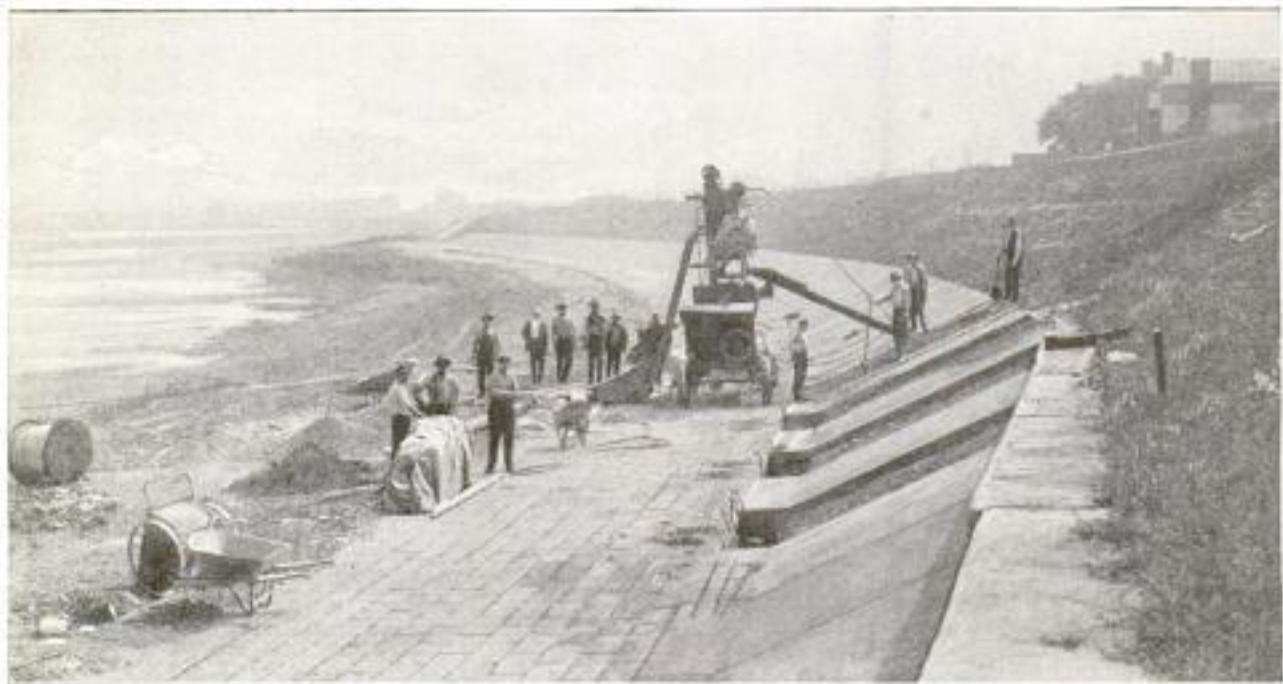
The Blocks are Anchored to Concrete Slabs Laid on the Bank just above them. The Tops of Piles, Driven at the Lower Ends of These Slabs, are Imbedded in Them When They are Poured, as are Also the Upper Ends of the Cables Which Run through the Blocks
