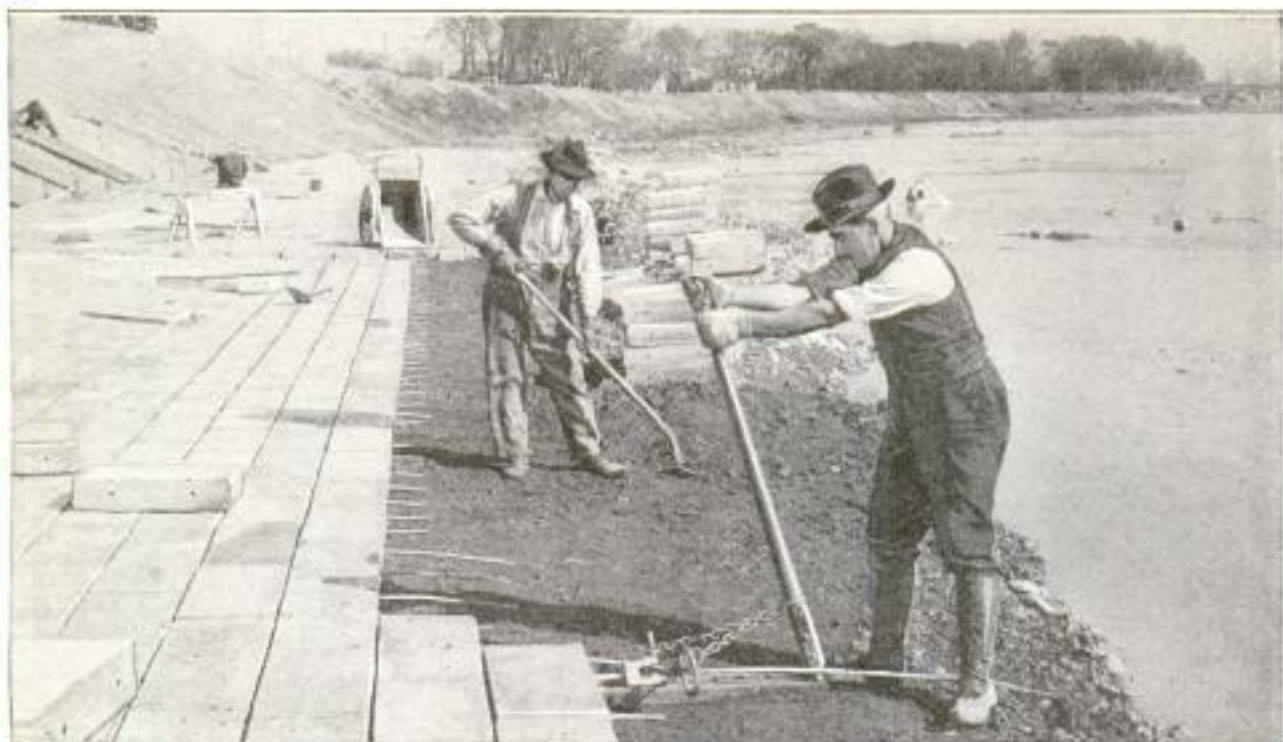
Laying Concrete-Block Paving along the Miami River at Dayton: The Ends of the Half-Inch Cables, Which Hold the Blocks in Place, can be Seen Projecting from the Last Row. Though the Cables Keep the Blocks from Sliding into the River, They Allow the Entire Mattress to Settle and Adjust Itself
