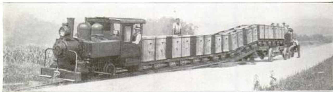
Train of "Batch Boxes," Used in Building This Cement Road, being Loaded, Three at a Time, on the Large Motor Truck at the End of the Inclined Track: These Batch Boxes are Then Transported, and Unloaded in a Similar Manner, Whereupon the Motor Truck Returns and Repeats the Operation
