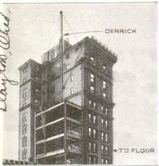
The Crane, Extending above the Tall Building, is Anchored to Its Wall. The Anchor can be Seen About Three Stories below the Roof
