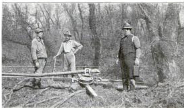
This Is the Hand-Power Stump Puller with Which the Donkey Engine was Hauled Out of the Swamp. The Lever Shown on the Mechanism Is 12 Feet Long
