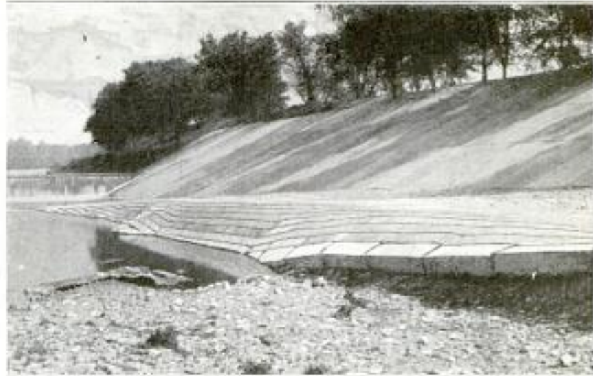
When Floods Scour Out the River Bed under the Edge of the Block Mattress, It Settles into the Depression. After One or Two Floods, the Mattress becomes Adjusted So That No Further Erosion and Settling Occur
