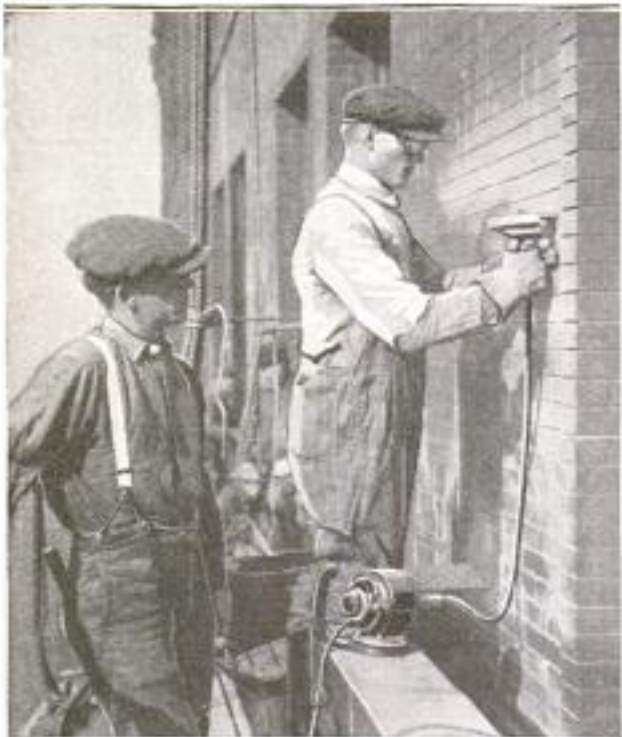
A Workman Removing Mortar between the Bricks of a Wall with the New Machine: Goggles Protect His Eyes from Flying Bits of Mortar
