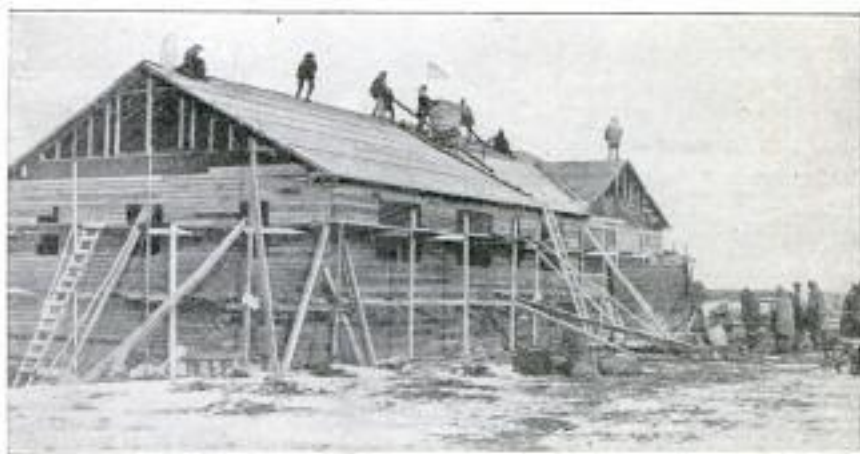
After the Frost Set In, the Chimney had to be Completed with Steaming-Hot Mortar. It Was a Source of Wonder to the Eskimos
