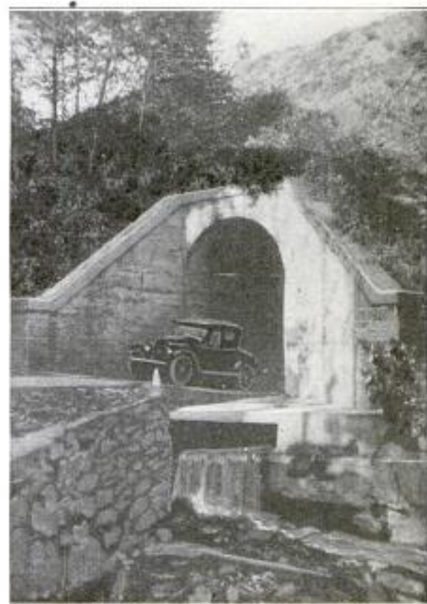
At the Top can be Seen the Railroad Right of Way; in the Center, the Automobile Demonstrates the Roadway, and at the Bottom, the Stream as It Is in Dry Weather
