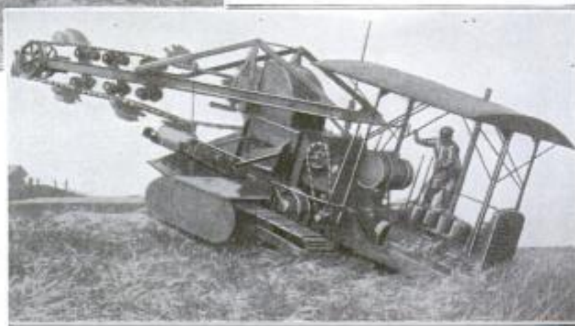
Trenching Machine Traveling over Rough Ground in War-Tank Fashion: The Digging Buckets are Seen on the Boom at the Rear
