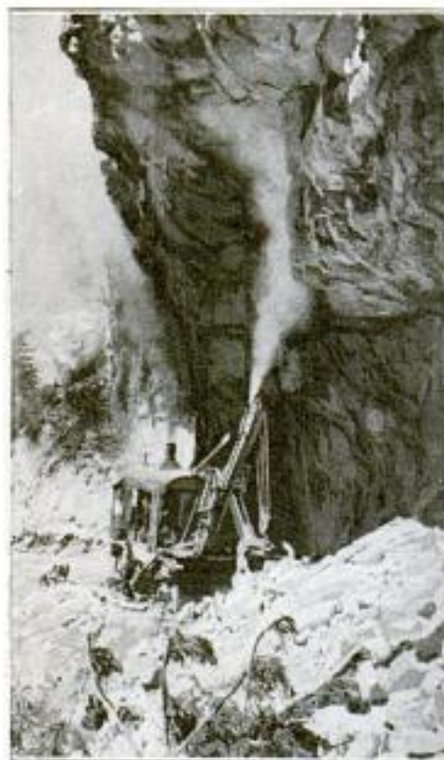
Steam Shovel at Work Cutting a Mile of Roadway along the Face of the Towering Cliff at Long Valley: Explosives Supplemented the Work of the Shovel
