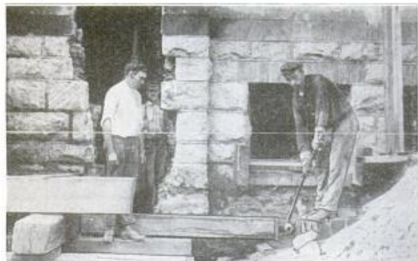
A Workman is Seen Here Operating One of the Jack Screws by Means of Which the "Slice" was Lifted for Moving
