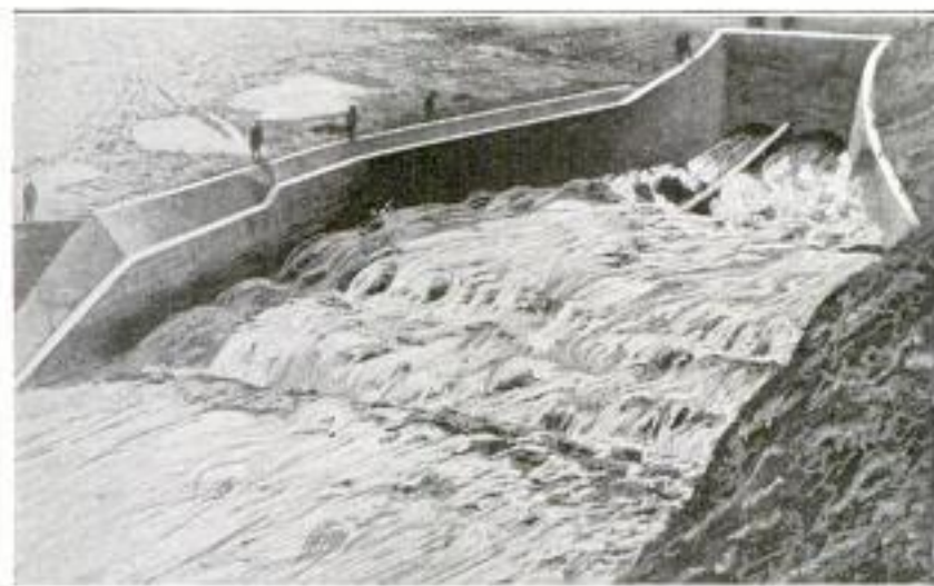
Outlet Conduits of the Germantown Dam, Showing How They Handled the Recent Flood: The Great Size of the Conduits is Indicated by Comparing Them with the Men Standing along the Far Wall
