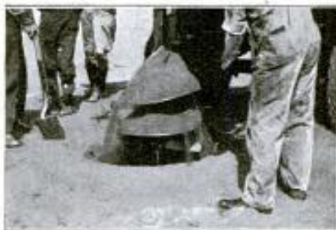
The Auger Bores Only a Little Way Down, and is Then Lifted Straight Up. Thus the Dirt is Lifted Out of the Hole, a Little at a Time, and the Boring Is Easier
