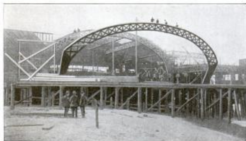
Lifting One of the 19-Ton Roof Trusses in Place in 40 Minutes by Means of an Electric Hoist
