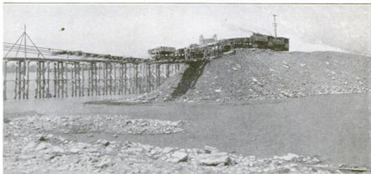
Making an Embankment across an Open Channel: Above the Light Trestle are Stretched Four Heavy Cables That Carry Railroad Ties, and the Rails onto Which the Cars are Backed and Then Dumped, So That There Is Never More Than One Loaded Car at a Time Unsupported by the Growing Embankment
