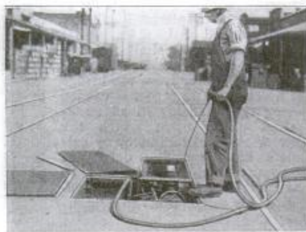
Air Hose and Compressed-Air Mechanism Used for Cleaning Switches in Oakland, California, in Connection with Electro-Pneumatic Switch Control
