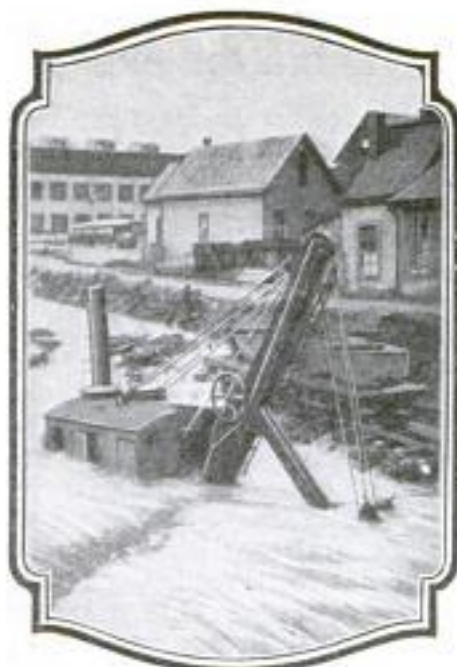
One of the Difficulties Encountered in Blasting and Dredging the Creek: A Sudden Rise in the Water Level Swamped This Excavator, and Put It Out of Commission
