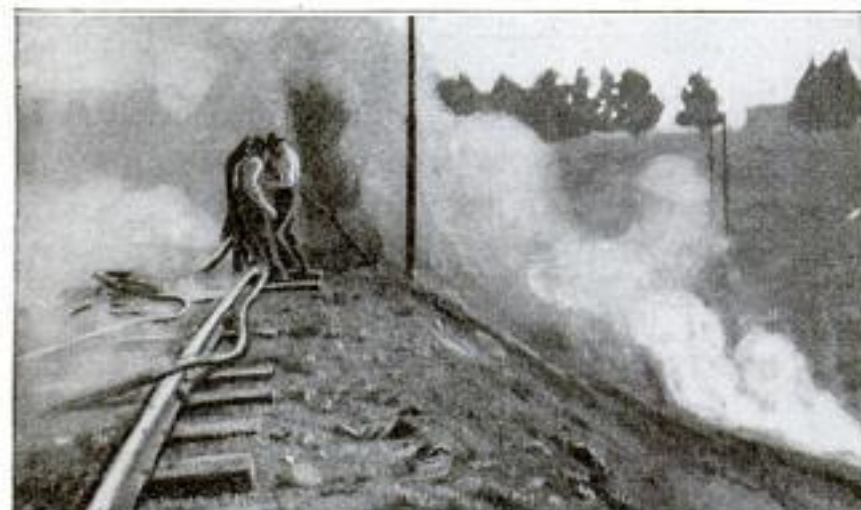
The Railway Embankment of Inflammable Material Is Ablaze, and the Fire is being Subdued with a Mixture of Baking Soda and Water Pumped through the Hose at High Pressure
