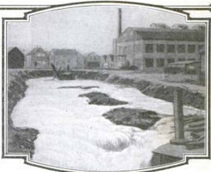
Part of the Creek being Prepared for Its Transformation into a City Sewer: The Dredge, Seen in the Foreground, was Submerged by a Sudden Rise of the Creek Water Level, and the Work could Not be Continued Until It had Subsided
