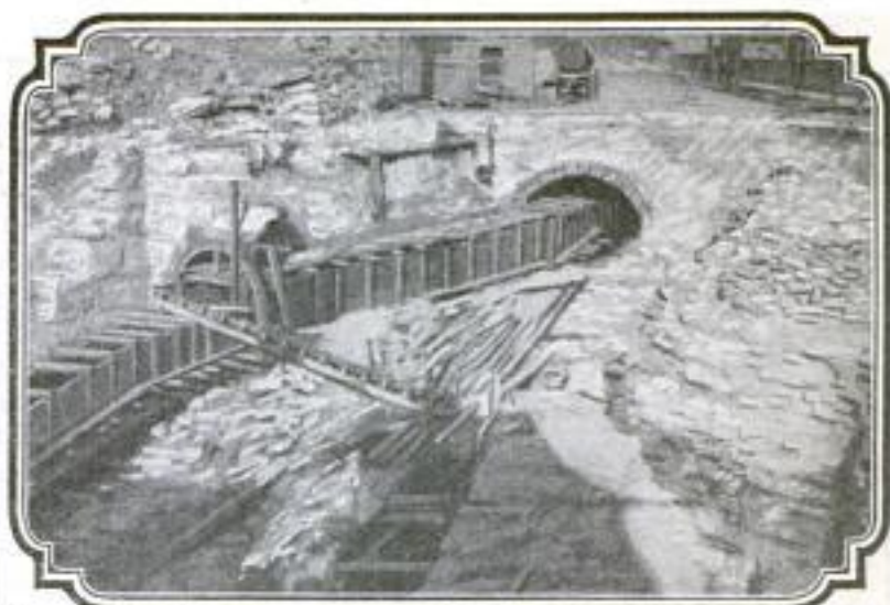
The Flume Which will Form a Sewer or Drain, Extending for Miles through the City of Buffalo, is Seen Partly in a Deep Excavation, and in the Background, Entering a Concrete Tunnel Which had to be Constructed for It
