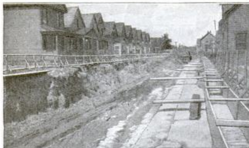
An Entire Street That had to be Excavated to Accommodate the New Drain or Sewer: This Condition of the Street Puts the Residents to Temporary Inconvenience, and Particularly Subjects Them to Danger in Case of Fire
