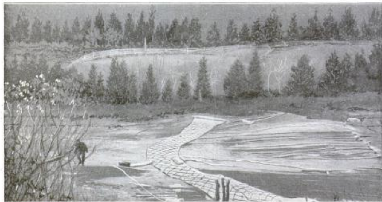
This Is the First Step in the Formation of a Temporary Dam across a Shallow Stream According to a System Devised in Norway. An Empty Canvas Hose is Laid across the Stream as Shown in the Center of the Picture
