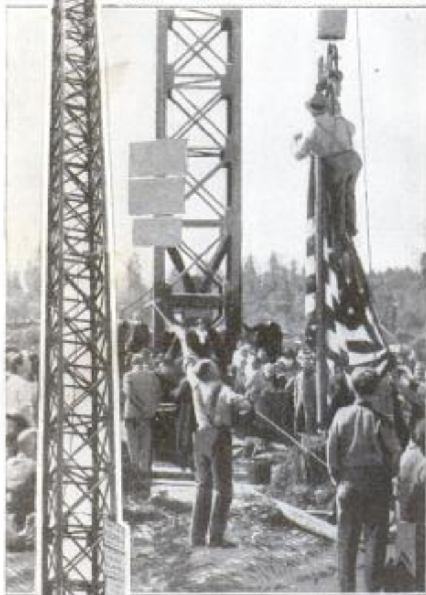
To the Left Is a Full-Length View of One of the Highest Wireless-Telegraph Towers on the Pacific Coast That was Recently Completed at Portland, Oregon. Above: the Men are Preparing the Flag to be Hoisted by the Mayor to the Top of the Tower During the Dedication Ceremonies
