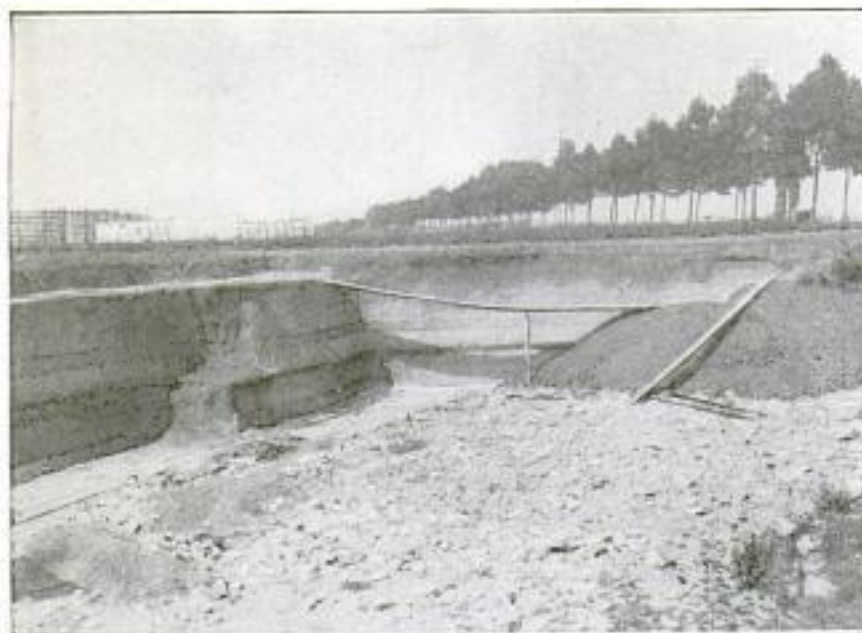
Working a Substratum of Gravel Out of a European Farm Field without Injuring the Crops: The Pile at the Right is Replaced Loam
