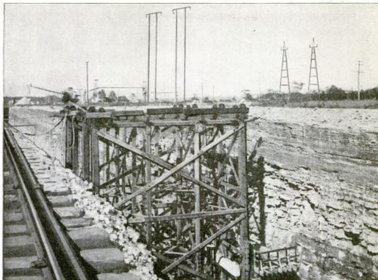
Finishing the Queenstown-Chippewa Canal around Niagara Falls: The Traveling Frame is Moved Along as the Work Progresses. One of the Suspended Platforms is Shown at the Right
