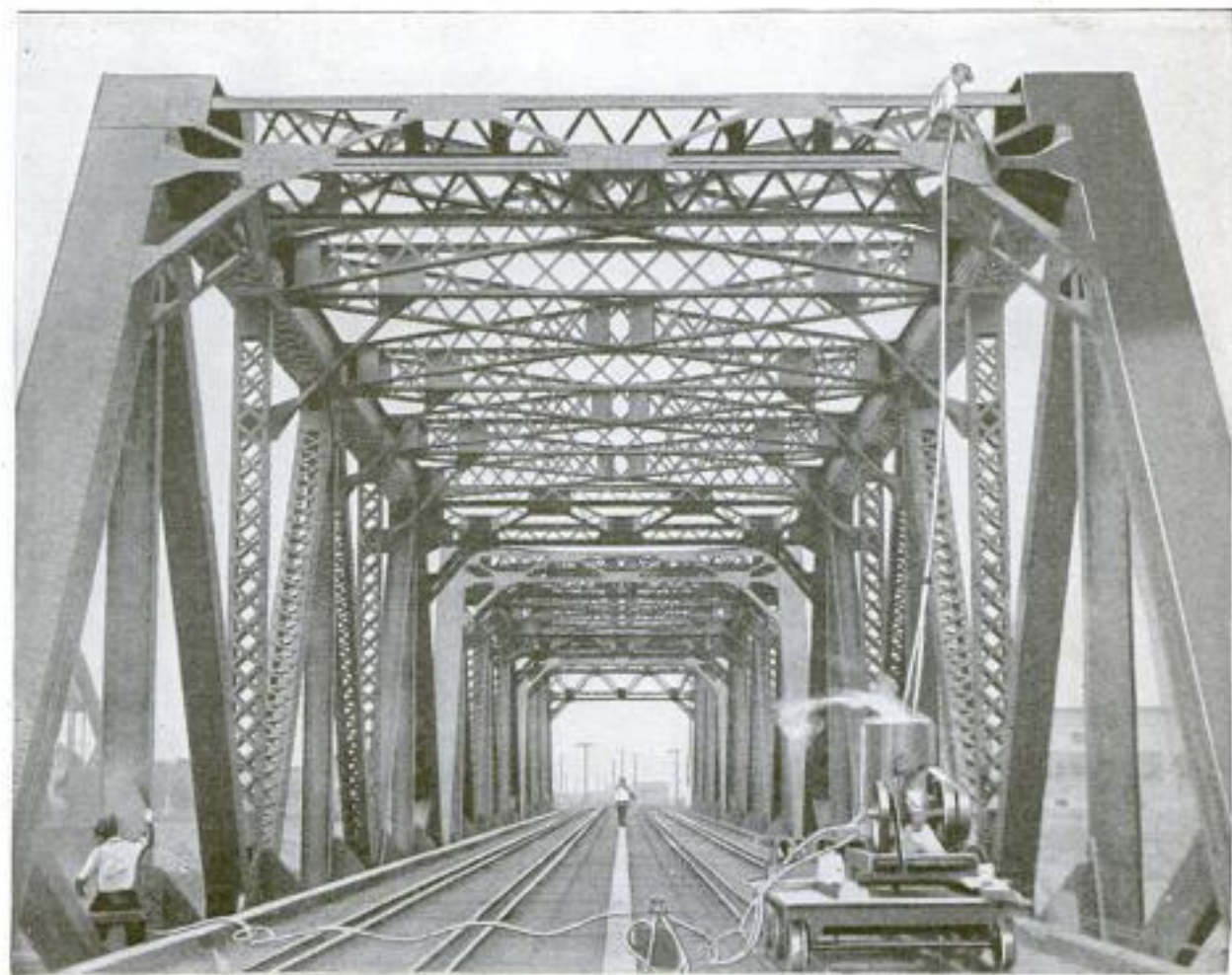
Using the Spray System of Painting on a Railroad Bridge, with the Aid of a Motor-Driven Car on Which the Air Compressor and the Tank for Paint and Air are Mounted: Two Paint Guns and Lines of Hose Assure a Rapid and Thorough Job of Coating the Intricate Ironwork
