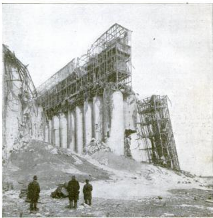
This Picture, Taken between the River and the Elevator, Shows How Some of the Storage Bins were Blown in Half, as the One on the Right
