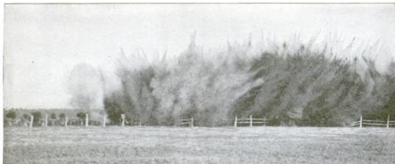
How the Acre of Stumps Looked When the Dynamite Went into Action: A Sufficient Amount of the Explosive was Placed under Each Stump and Connected by Wiring. An Electric Impulse was Transmitted to All Simultaneously
