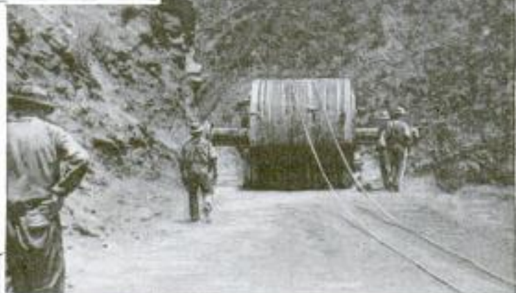
Narrow Uphill Passes Were Some of the Difficulties Overcome. The Picture Shows a Rotor Passing through One of Them. The Cables in Front are the Pulling Lines
