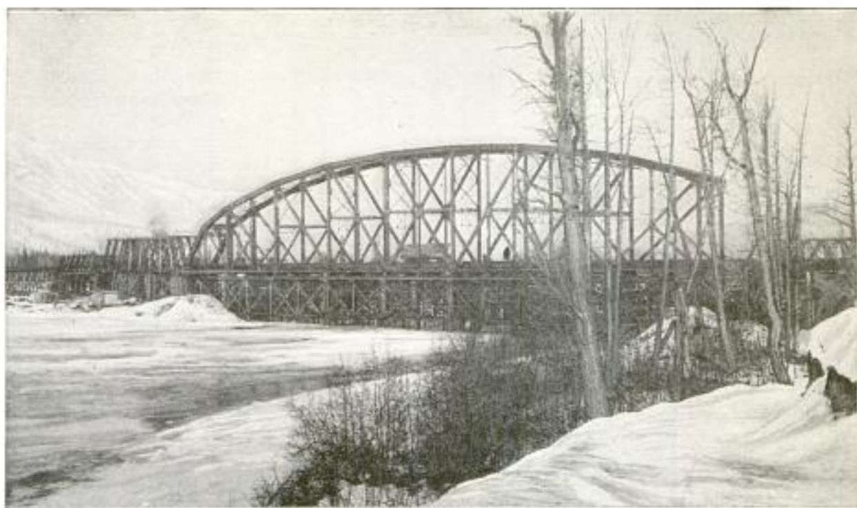
A View Taken Just before Christmas, 1920: The Susitna River Bridge under Construction during an Alaskan Winter, with the Steelwork Nearly Completed. The Picture was Taken Looking West, and Downstream.
