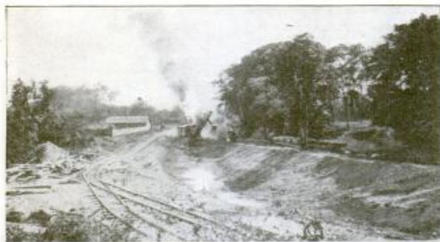
The Excavator at Work, Deepening the Channel of Onondaga Creek at Syracuse, and Preparing Its Bed for the Concrete Lining
