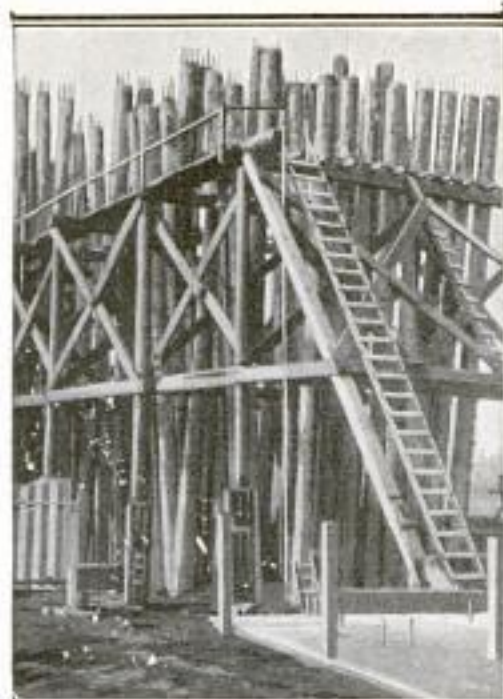
Finished Piling Standing in the Curing Frame, Where It is Allowed to Remain for 30 Days, and is Sprayed with Water Every Day
