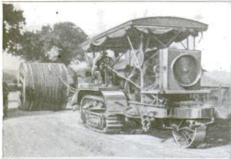
Unwinding Cables Pulled by a Caterpillar Tractor, Rolled the Giant Rotors over a Mountain Road to the Power Station. Two 750-Foot Cables and Two Tractors were Used for the Job
