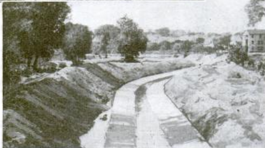
The Finished Concrete Floor, 28 Feet Wide, Ready for the Construction of the Side Walls on the Sloping Earth Banks
