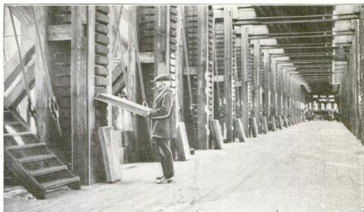
The Railroad or Wagon Bed of the Pontoon Bridge Rests on Cribbing Piers. Blocks in the Piers are Removed or So Placed as to Keep the Roadbed on a Constant Level. Machinery Holds the Bed Up While the Blocks are Changed
