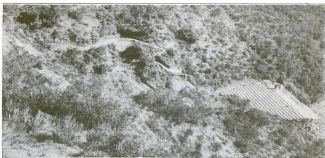
Early Stages of the Construction Work on "The Pilgrimage Play" Stadium in the Cañon: At the Right, Workmen are Seen Building the Scaffolding for the Seats, While the Site of the Stage at the Left is Concealed in the Ravine. More than 200 Players Appear in the Production
