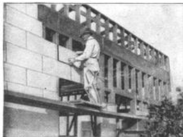
The Concrete Slabs are Used in Place of Lath, and Have the Appearance of Gigantic Bricks. The Method of Application is Shown Here
