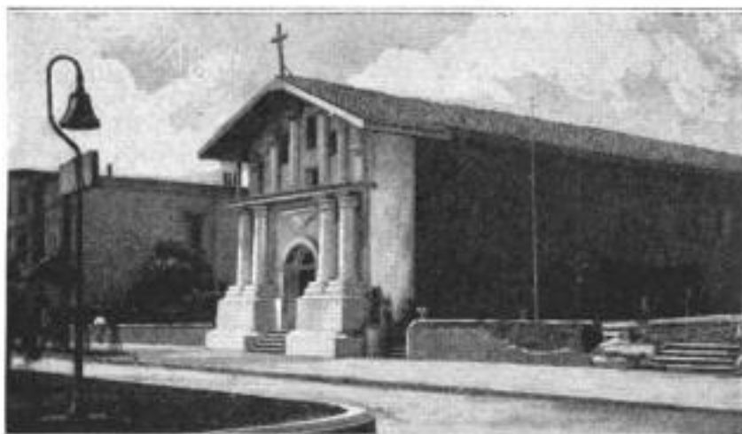
The Crumbling Adobe Front of This Ancient California Mission was Reinforced, Recently, with Concrete. This Is Doubtless the Most Extensive Repair Made in the Church's Century and a Half of Existence
