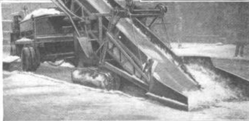
Five-Ton Trucks, Fitted with Sideboards to Increase Their Capacity, were Filled in an Average of Five Minutes Each by the Snow Loader
