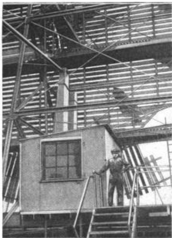
View of the Back of the Big Clock, Showing the Method of Diminishing Its Resistance to the Wind: An Electrically Controlled Driving Mechanism of Unusual Power is Housed in the Shed
