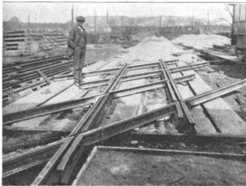
Thermite Welding of Railway-Crossing Frogs is being Used Extensively. The Joints will Not Loosen from Vibration as Do the Bolted Type
