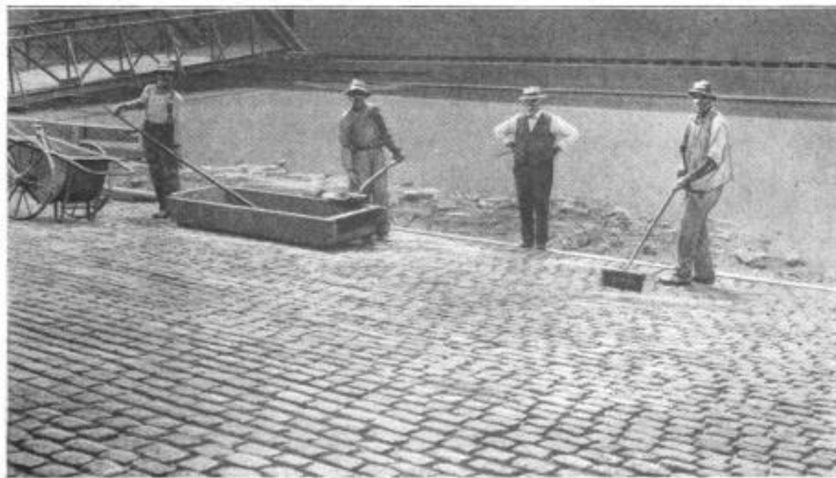
Cincinnati's New Public-Wharf Approach is Calculated to Withstand the Ravages Incident to the High-Water Periods. Mud, Settling in the Wide Interblock Spaces, is Easily Flushed Out. The Wide Spacing Also Affords a Good Foothold for Horses
