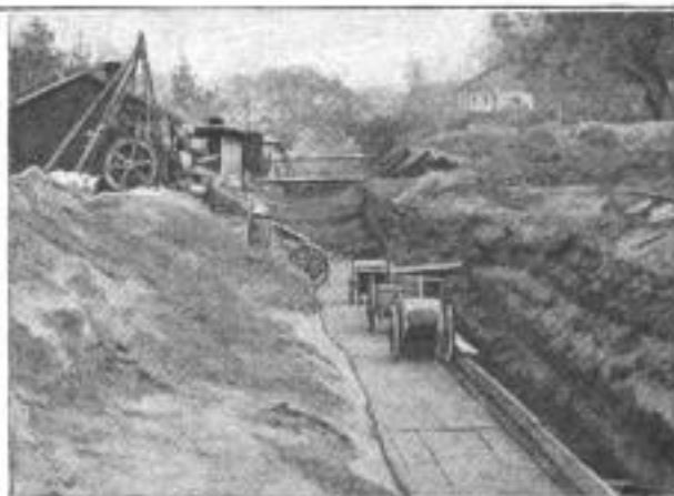
Ready to Pour the Cover: After the Concrete had Hardened, the Planking and Steel Pipe were Removed and the Cover Dropped into Place
