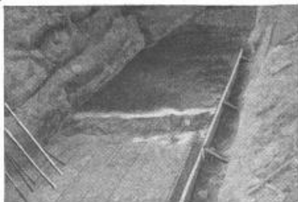
A Finished Section: All That Remains Is to Remove the Planks and Lower the Cover into Position, Sealing the Top Opening
