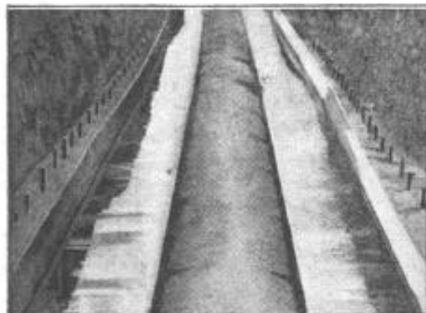
Here is Shown How the Concrete Conduit was Cast around the Old Steel One, Leaving Only Space Enough for the Removal of the Latter
