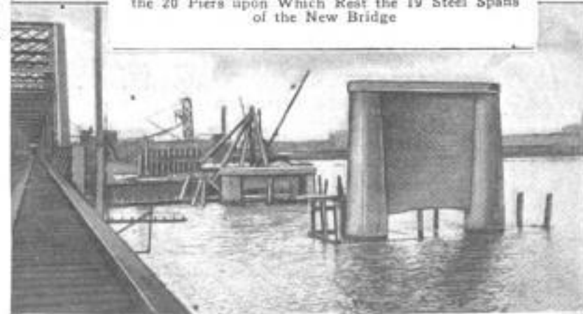
The Approach and First Pier at the Jacksonville End of the New Bridge. Proximity to the Railway Bridge Necessitated Some Adroit Engineering at One Point, to Avoid Interference with Its Swinging Span
