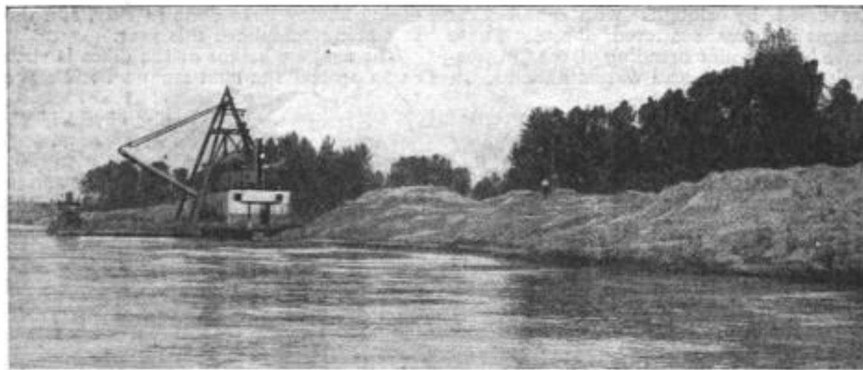
One of the New Dikes under Construction in the Multnomah District: The Work is Done by the Big Barge at the Left, Which Takes the Material from the Dredges, Brings It to the Dike Location, and Dumps It
