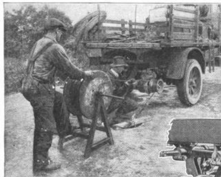
An Underslung Motor-Truck Power Winch Driven by the Engine, Pulling Telephone Cables through Street Conduits: Should the Insulated Cable Meet with an Obstruction, the "Feel" of the Off-Coming Power Cable Warns the Operator to Ease the Pull
