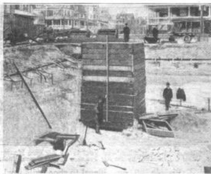
The Box Test for Building Foundations on Sand: Loaded with Rock. It Exerts a Pressure of Six Tons to the Square Foot, or Twice the Load of the Finished Building
