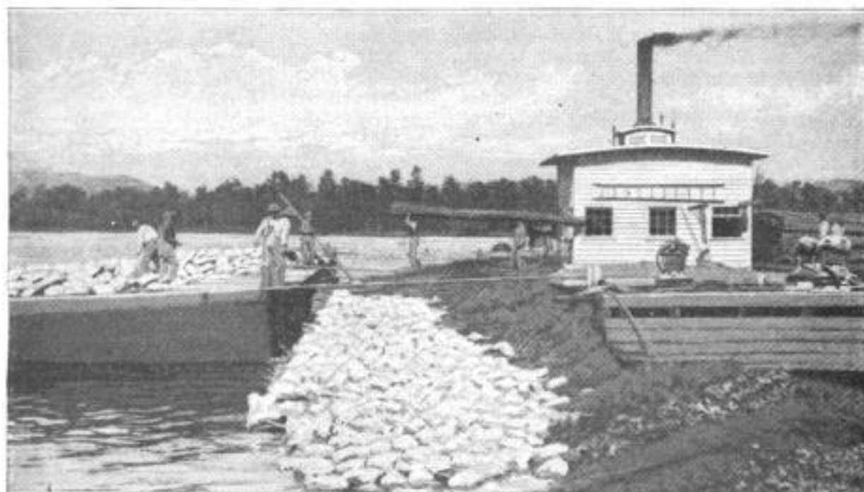
The Floating Power House Used in the Work of Straightening the Mississippi River Channel: The Barge of Rock is Seen at the Left, and the Load of Willow Mattresses at the Right, behind the Power House, from Which Both are Controlled by Winches and Cables on the Deck
