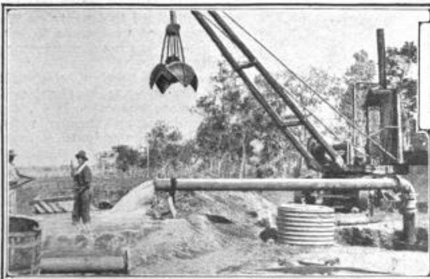
The Orange-Peel Type of Grab Bucket was Used in Excavating for the Well Cylinders, as at the Left. The Large Output of the Wells is Indicated by the Stream of Water Drawn by a Test Pump from a Five-Foot Bore in the Right Foreground
