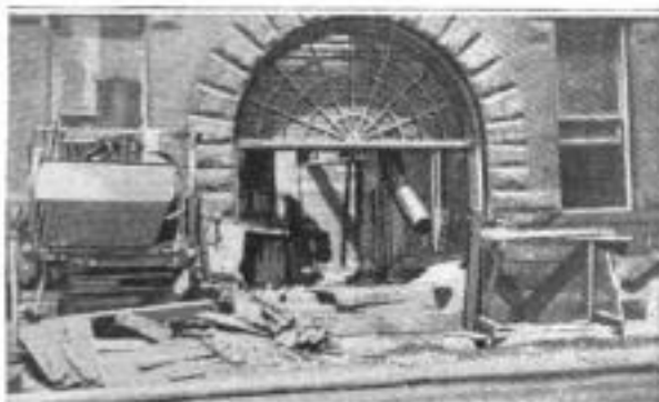
A Quantity of Large-Diameter Tin Pipe, Connected to Make a Chute from the Upper Floors of a Remodeled Building, Enabled the Contractor to Remove the Débris Conveniently
