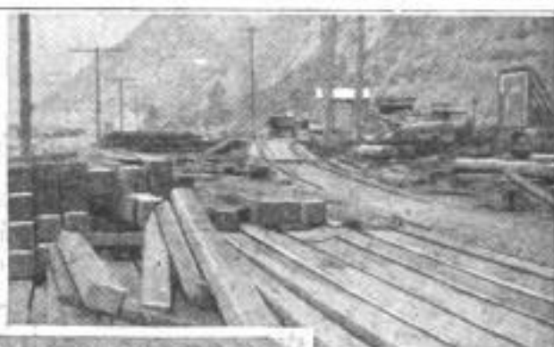
The Improvised Plant on the Beach, Where the Old Piles are Cleaned and Coated with Preservative
