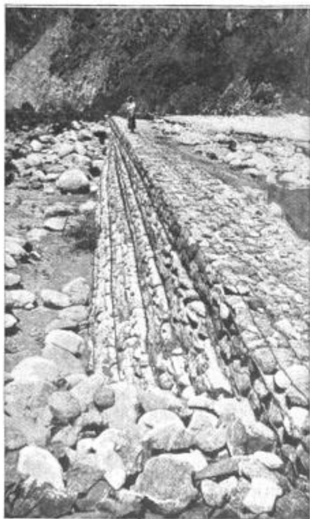
Close Inspection of This River Dike Shows That the Stones are Held in Place by Netting of Heavy Wire. The Five Courses can be Distinguished
