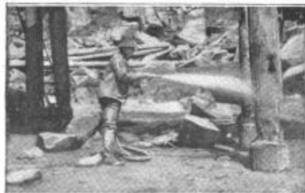
Using a Cement Gun to Place a Protective Coating of Sand and Cement on Old Wood Piling
