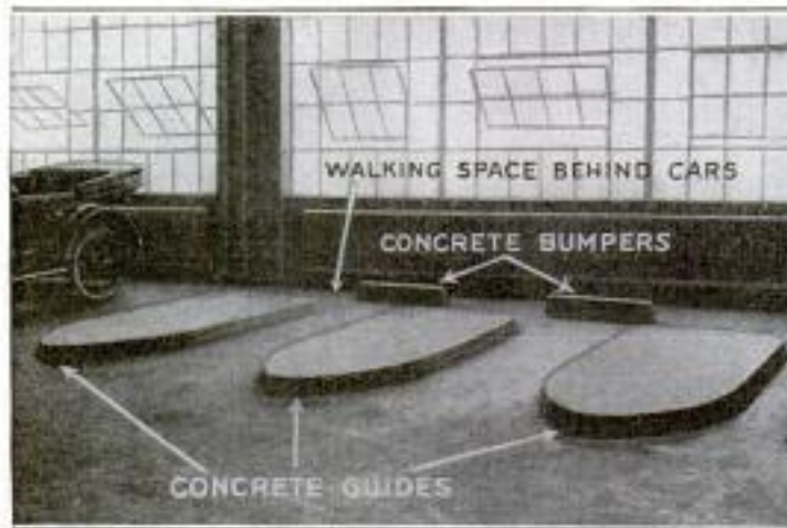
A View of the Safety Platforms That Prevent Careless Drivers from Colliding with Other Cars: At the Back of Each Stall Are Concrete Bumpers
