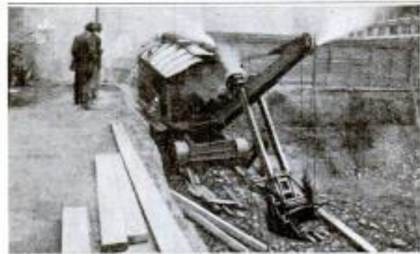
Steam Shovel Pushing Itself Out of an Excavation: The Jets of Escaping Steam Show That the Machine is Prepared for Maximum Effort
