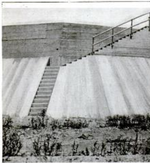
The Steps in This River Wall Enable Pedestrians to Cross the River Bed at This Point during the Dry Season Instead of Walking Several Blocks to a Bridge
