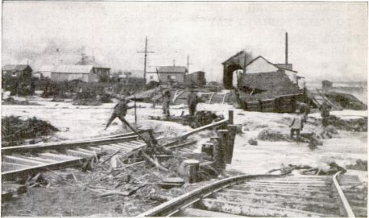
One of the Points at Seward, Alaska, Where the Government's New Railway Line was Washed Out by the Raging Torrents That Swept through the City
